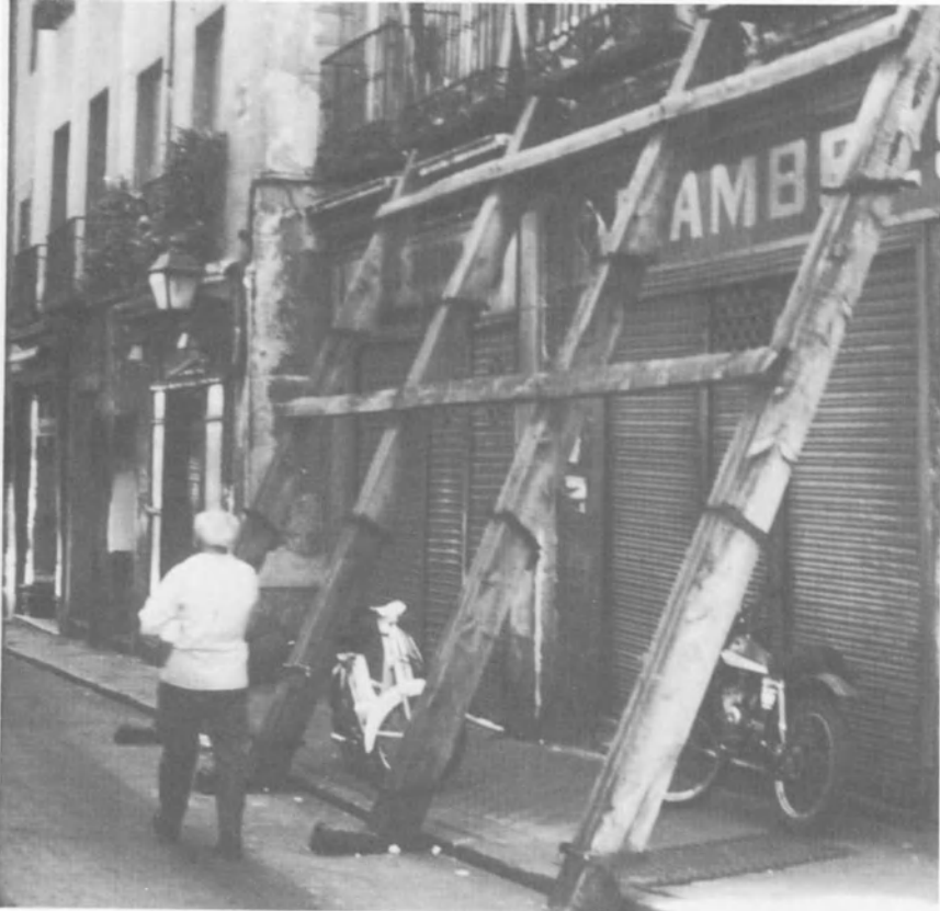
Figure 8. La Corrala. Like many other buildings in the neighborhood, this one was declared “in ruins” and boarded up.
