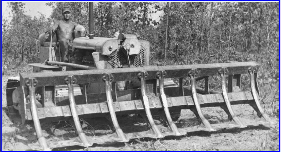
Figure 5.20 Site preparation machinery. Root rakes windrow brush and weed trees prior to planting and direct seeding operations.
