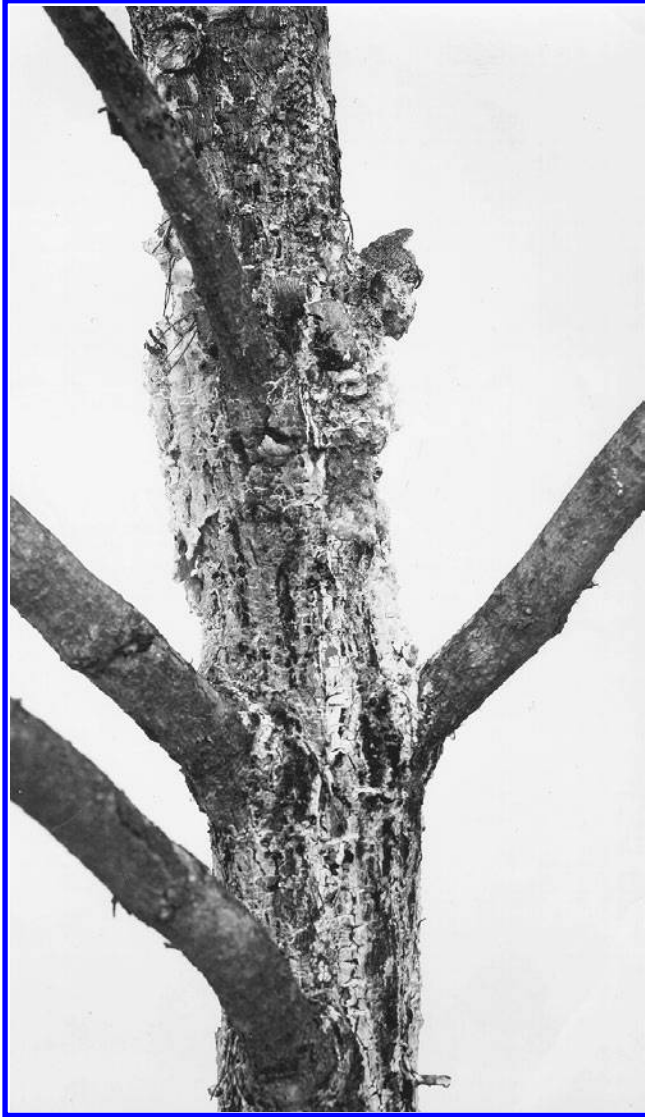
Figure 6.16 Pitch canker on Virginia pine, caused by Fusarium lateritium . The tree is alive below and dead above the infection site. Trunk cankers develop on trees of any size, spreading until the trunk is girdled, the tree dies, or is broken off. (USDA Forest Service photo by G. Hepting)
