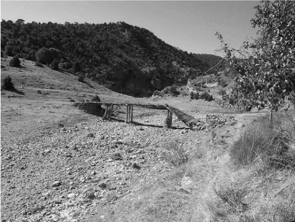
Figure 4.14 Ruined wooden bridge near Han Derbent, at the eastern end of the Kûfû Vadisi (the western fringe of the plain of Sandıklı)
