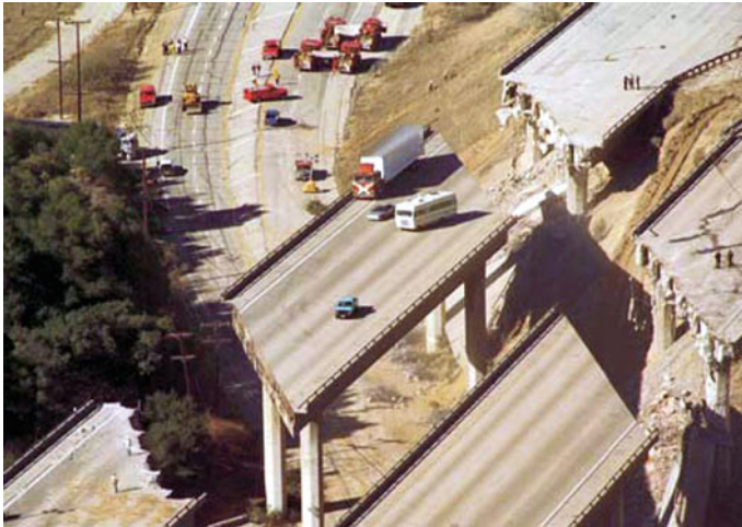
Fig. 1.4 Bridge collapse during an earthquake at Northridge in 1994, USA
