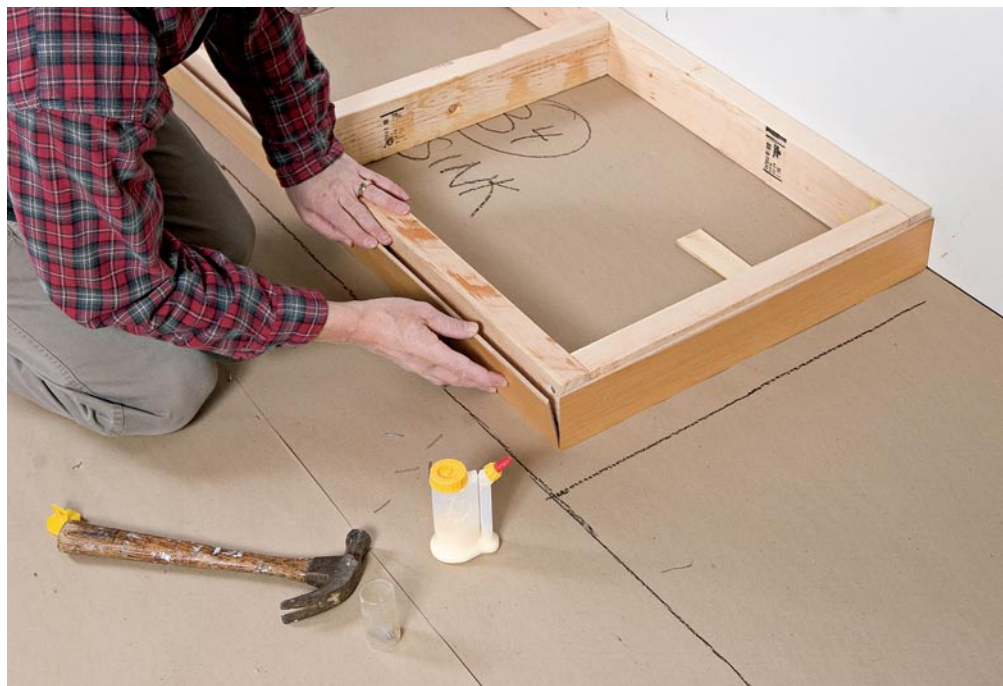
With the base frame secured, I then apply prefinished strips of 1/4-in. plywood veneer to the exposed faces.
