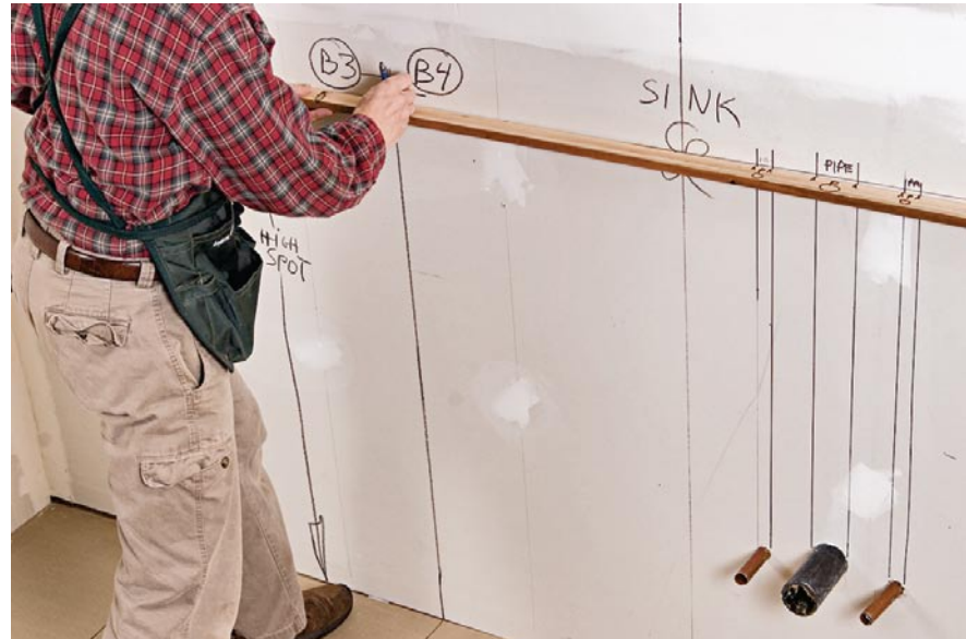
Here I'm transferring the intersection points to the story pole held to the reference line.
