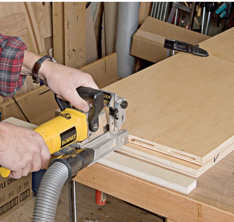
With the spline-biscuit joiner centered on the layout marks on the edge of the floor panel, I cut the slots from right to left. Note the scrap of case plywood used to support the base of the tool.
