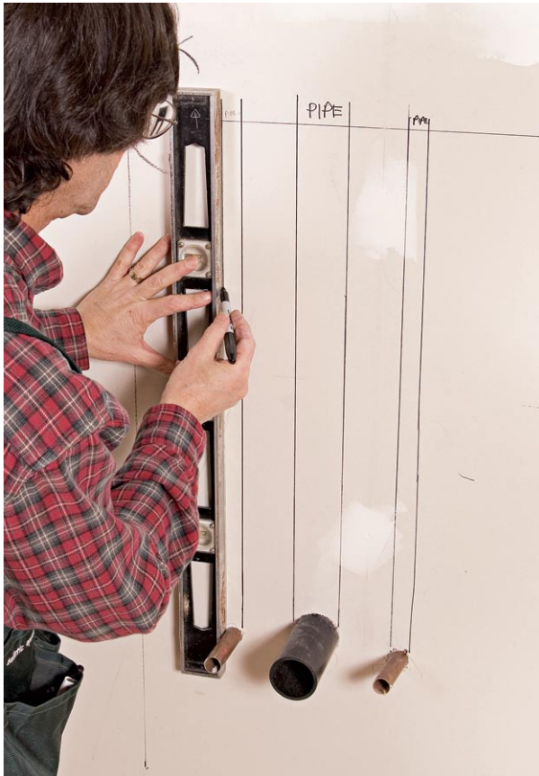
Using a 30-in. bubble level, I draw plumb lines from the pipes to the reference lines.
