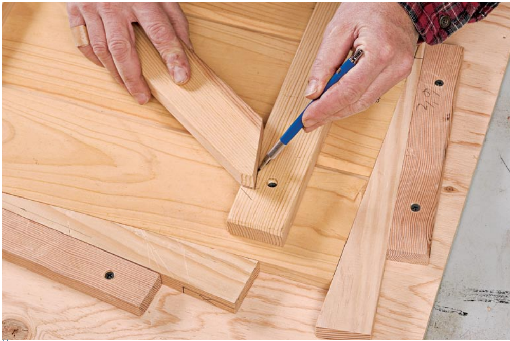
As an alternative to using the standard Z-brace, I extend the ends of the diagonal brace into the cross battens, producing a shouldered Z-brace.
