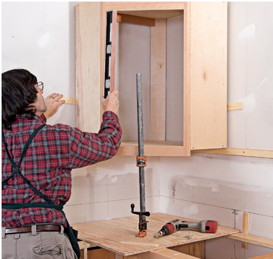
I begin the installation of a run of upper cabinets with a corner unit. Here I'm adjusting the face of the unit plumb while it sits on its ledger. The pipe clamp (with a reversed head) prevents the cabinet from pitching forward.
