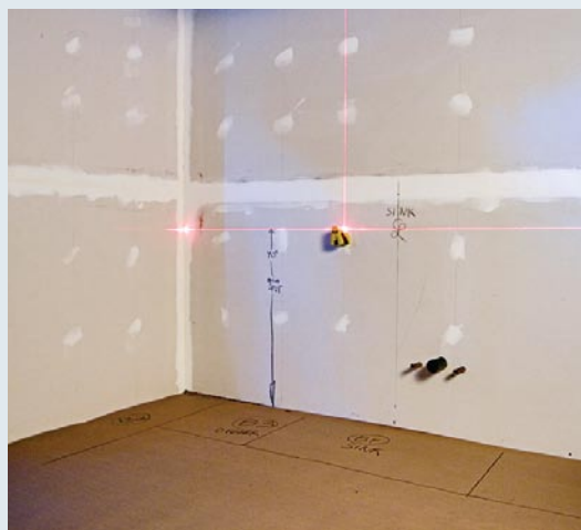
An inexpensive, self-leveling laser level—held to the wall with double-stick tape—shoots a line along the surface to create a reference line.
