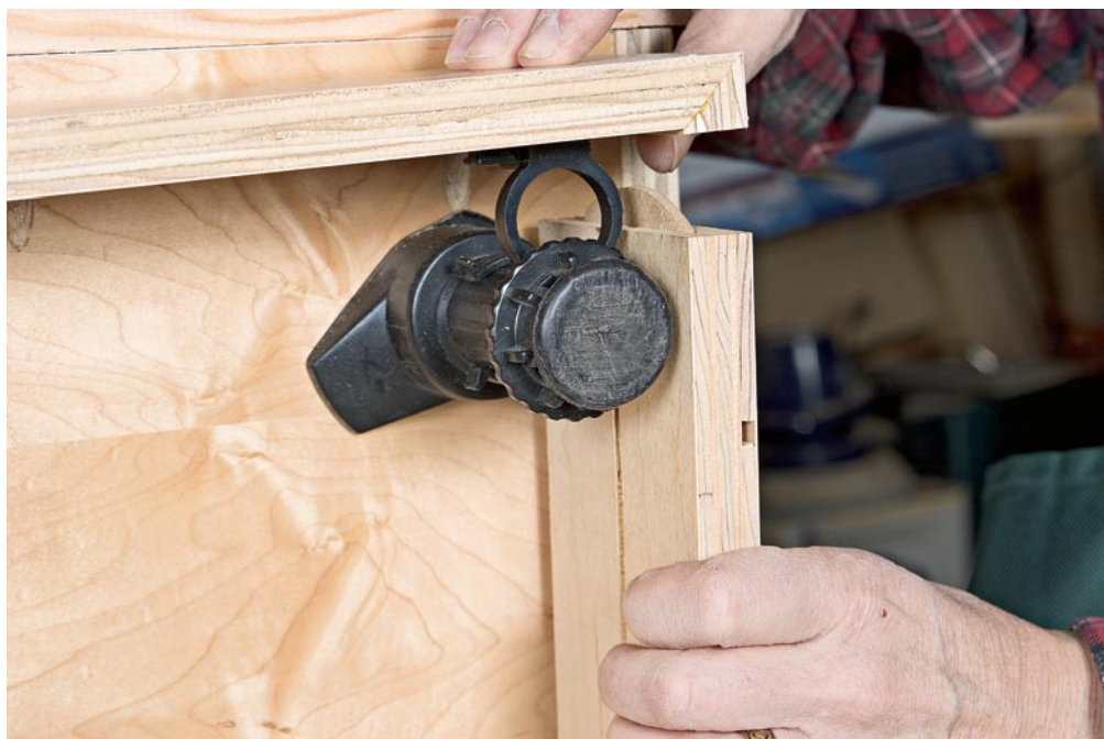
To install the kick boards, I press the clips over the adjustable leg levelers. Note the spline biscuit, which helps keep the corner in alignment.
