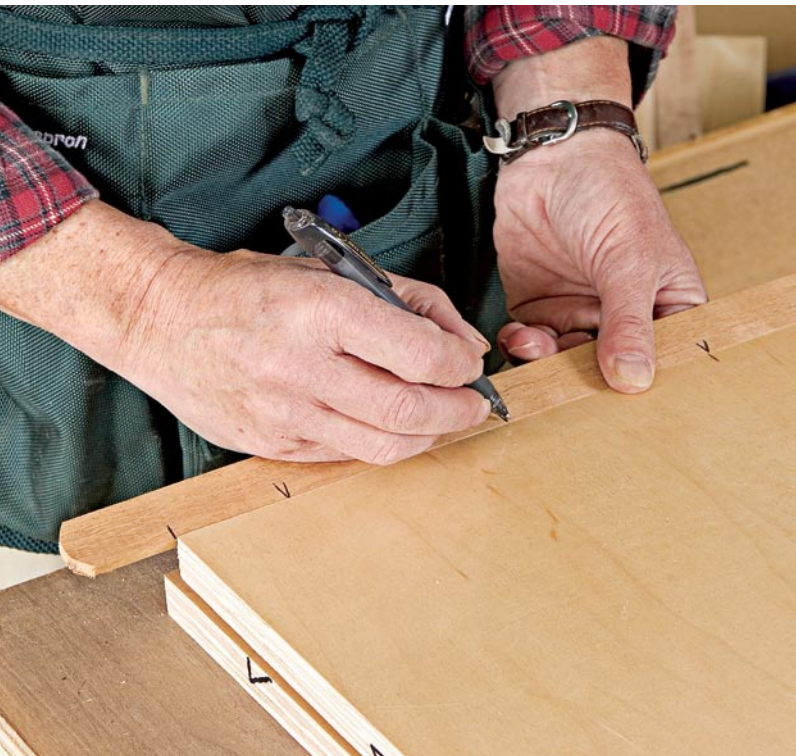
A marked stick speeds up the process of laying out the slots for the spline biscuits on the floor panel.
