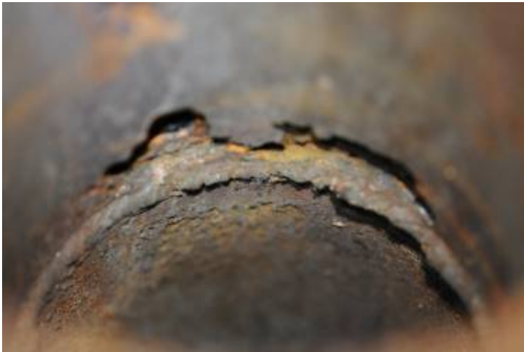
Figure 15. An excessive overfill and severe surface degradation beside overfill at 6 o'clock position.
