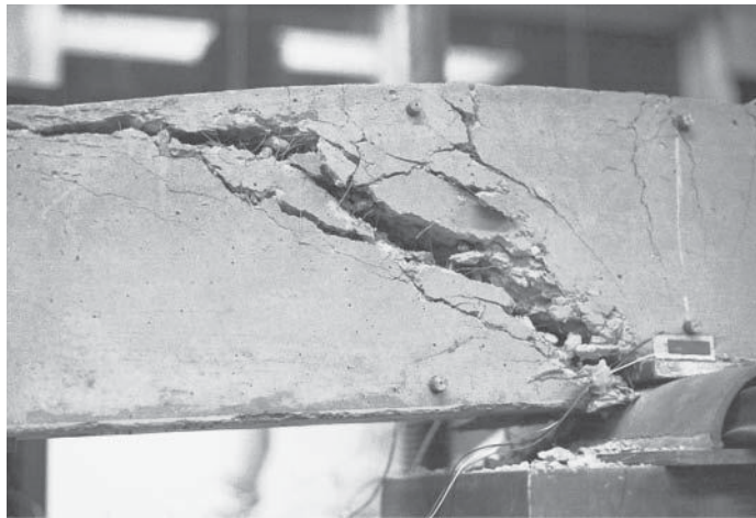
Shear failure near a middle support.
