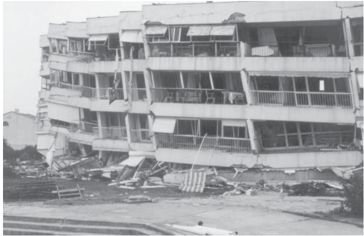
Collapse of frame concrete structures due to an earthquake. Courtesy of Murat Saatcioglu and John Gardner.
