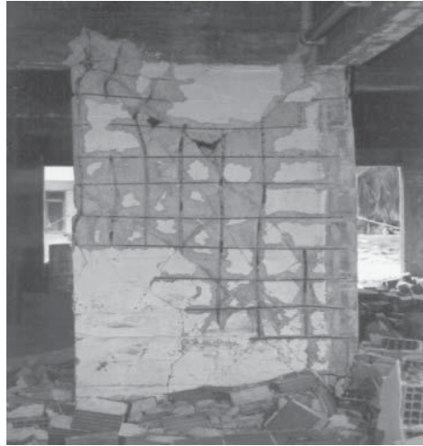
Shear wall after an earthquake. Courtesy of Murat Saatcioglu and John Gardner
