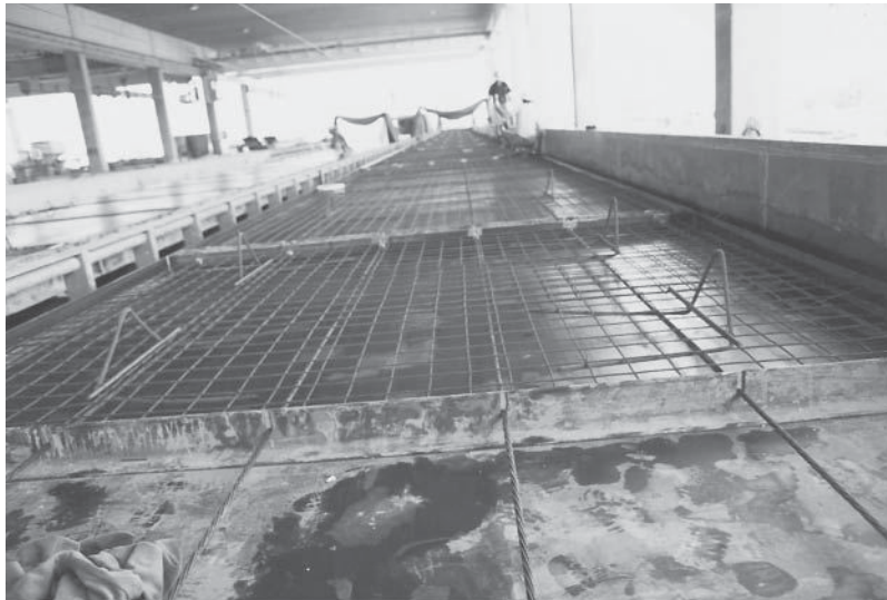
Prestressed concrete beds for slabs and wall panels.
