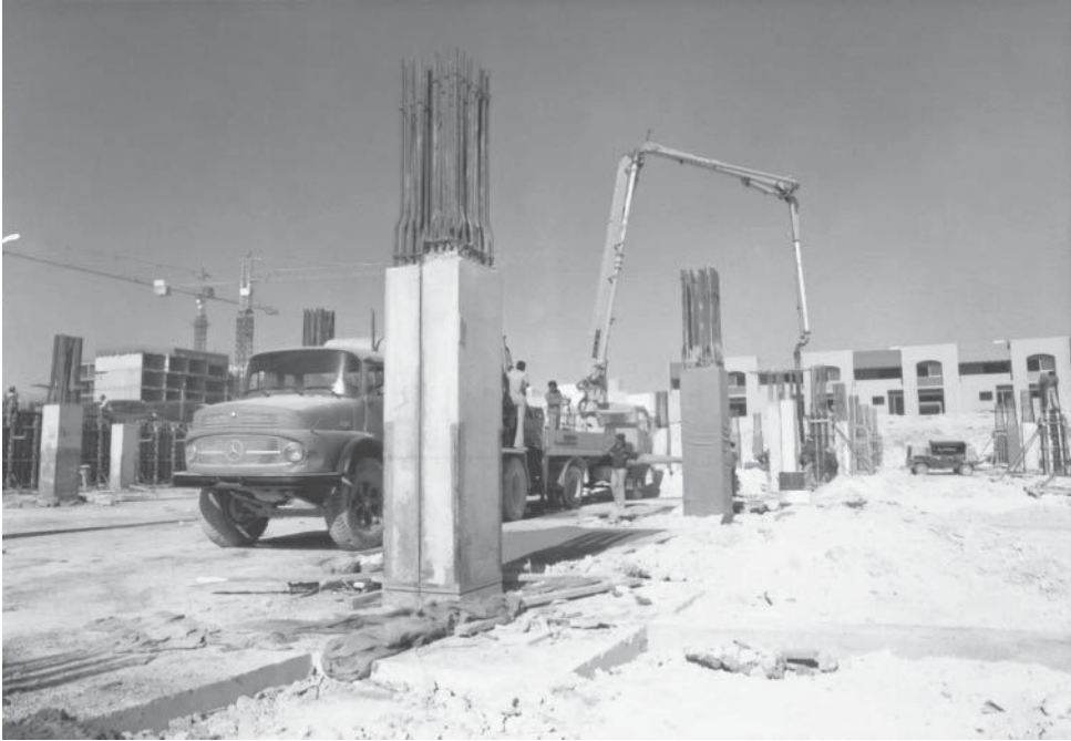
Reinforced concrete tied column under construction. The two columns are separated by an expansion joint.
