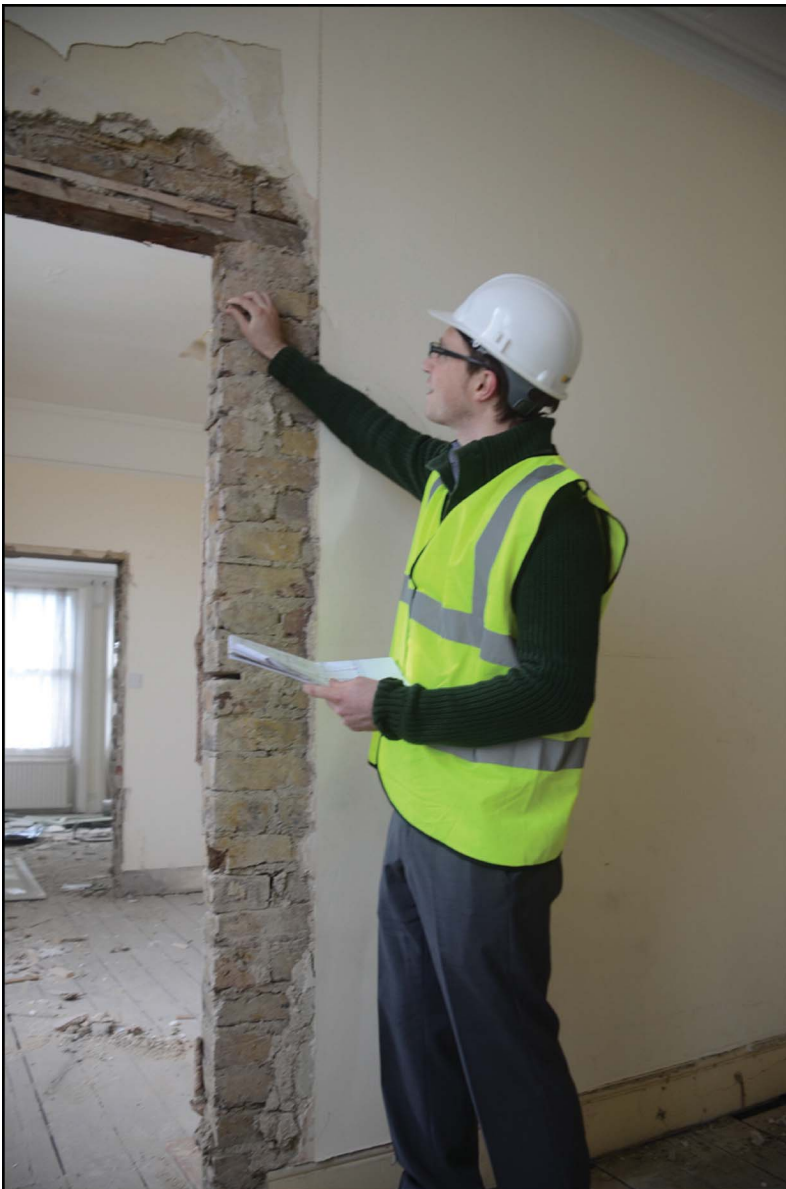
Figure 17 As well as working on designs, structural engineers often work on appraising the nature and condition of the structures of existing buildings
