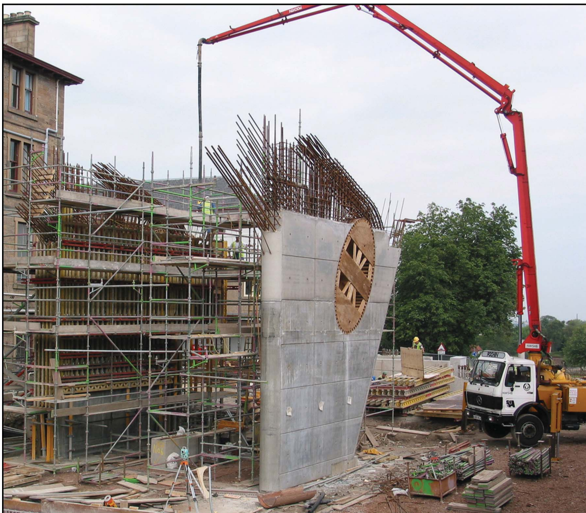
Figure 15 This example of reinforced concrete construction is for a lecture theatre in Edinburgh. The combination of many decisions made by different design disciplines are integrated into the construction of the finished product
