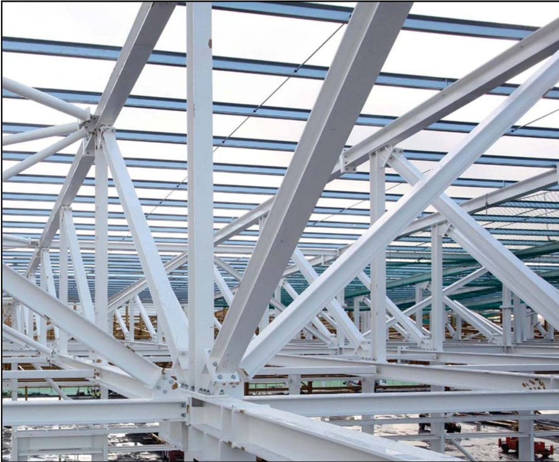
Figure 11 Steelwork structure – completion of the design of connections may be undertaken by the constructor
