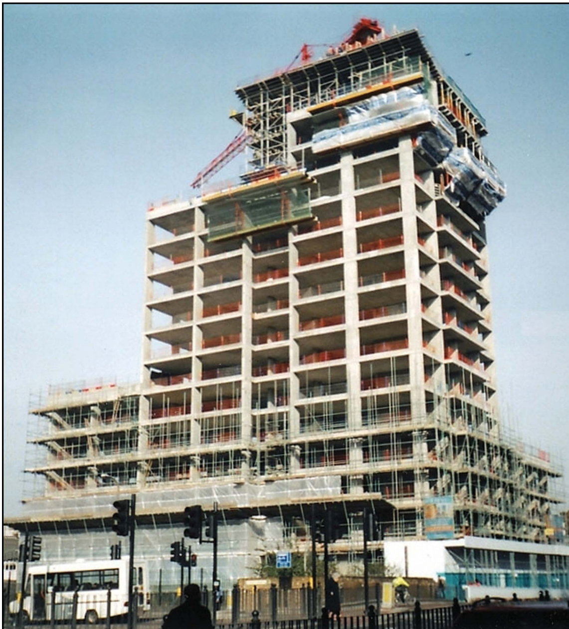
Figure 13 A reinforced concrete framed apartment block under construction in East London. A building such as this could be procured by one of a number of different approaches
