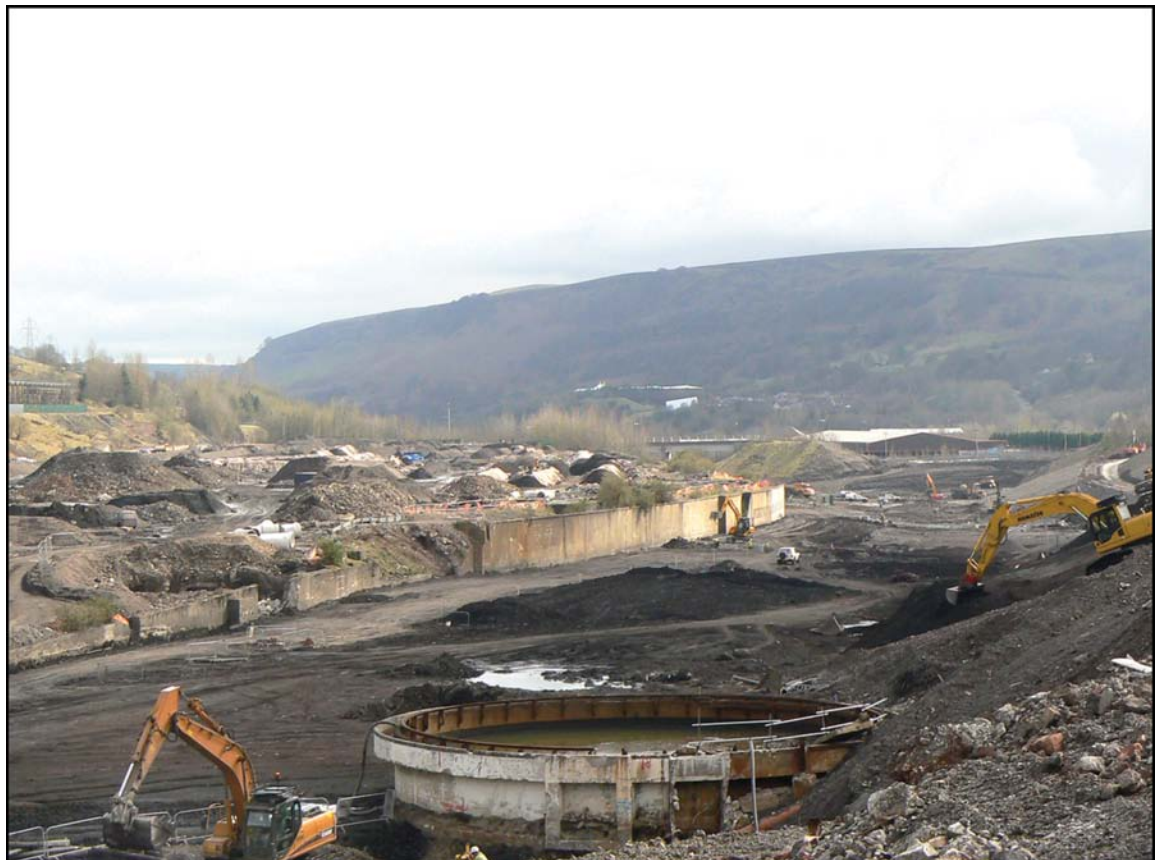
Figure 5 As this former steelworks site is cleared, formerly hidden features become exposed and any contamination in the soil can be identified
