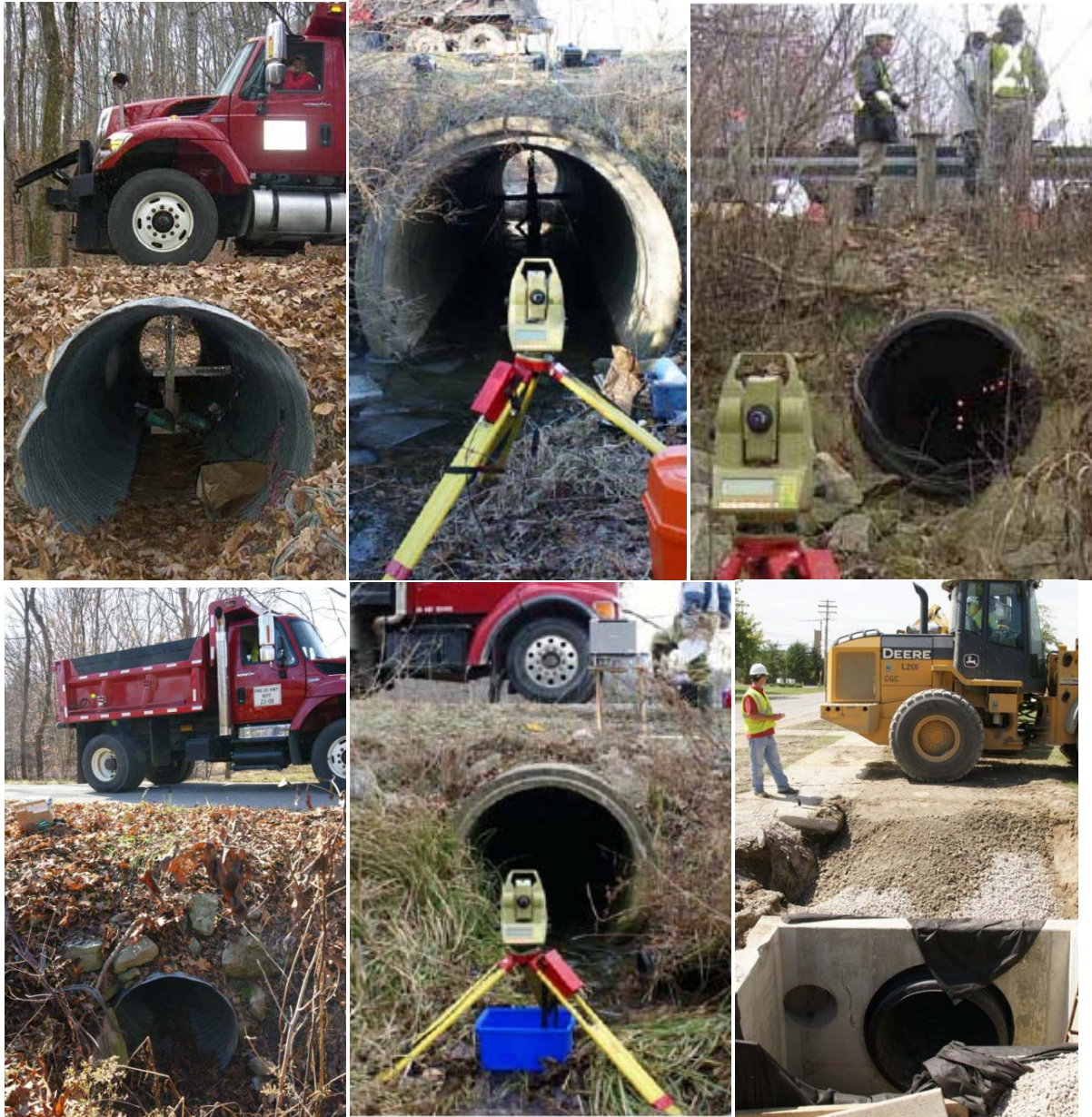
Top left (first CSP), Top Middle (first RCP), Top right (first HDPE pipe) Bottom left (second CSP) Middle (second RCP), Bottom Right (second HDPE pipe). Figure 1 Images of the six culverts in Ohio tested under vehicle loads.
