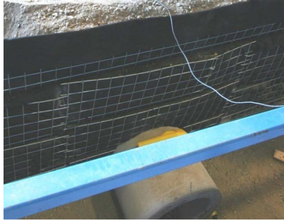
Figure C.15. Grid with Geosynthetic used for the end-wall treatment for all burial testing (shown here with 4ft of cover soil over the 24 in diameter specimen).
