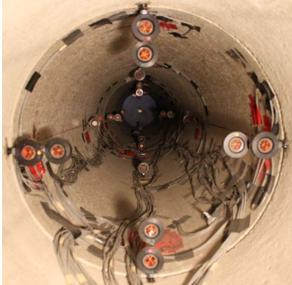
Figure C.9. View of the prisms after placement in the 24 in (610mm) diameter reinforced concrete pipe.
