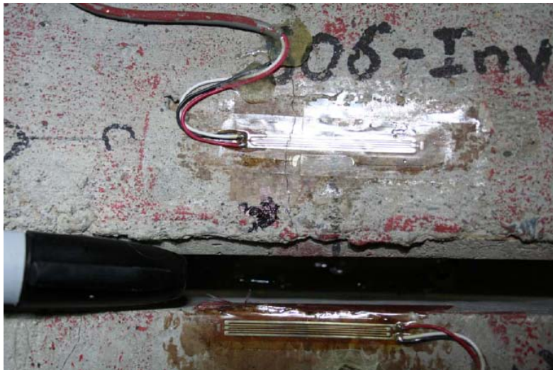
Figure C.26. Close-up of the invert of the 24 in. (610mm) diameter reinforced concrete pipe at the central joint; the joint is open about 1 in (25mm).
