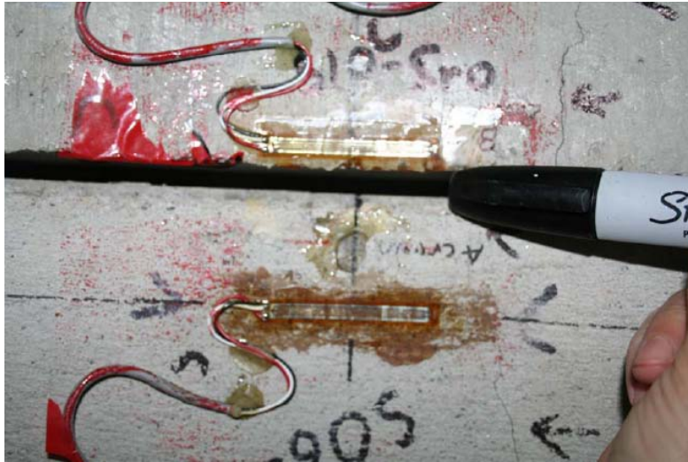
Figure C.27. Close-up of the crown of the 24 in. (610mm) diameter reinforced concrete pipe at the central joint; joint open about 0.5 in (12.5mm).
