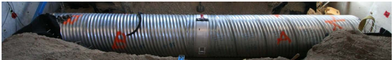
b. 36 inch (914mm) diameter corrugated steel pipe with unsealed band joint
