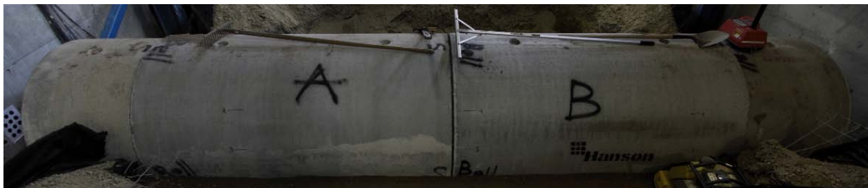
e. 48 inch (1.2 m) diameter reinforced concrete pipe with unsealed bell and spigot joint
