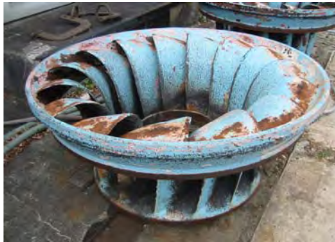
Fig. 2. Cavitation erosion on the old runner.
