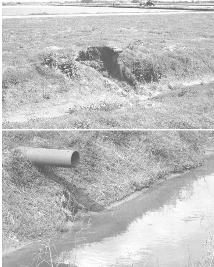
Fig. 6.6. Improper and proper installation of embankment pond drains. Erosion around the improperly installed drain (top) has washed approximately 5 m 3 of soil into the receiving stream. The properly installed drain (bottom) extends beyond the foot of the embankment into the receiving stream. Photographs courtesy of Danny Oberle.
