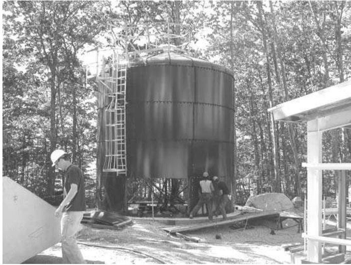
Fig. 10.12. A biosolids storage tank, such as this one at the United States Department of Agriculture, Agricultural Research Service, National Cold Water Marine Aquaculture Center in Franklin, Maine, is designed to hold months of captured and thickened biosolids with no discharge until the stored biosolids can be hauled to a final disposal site.
