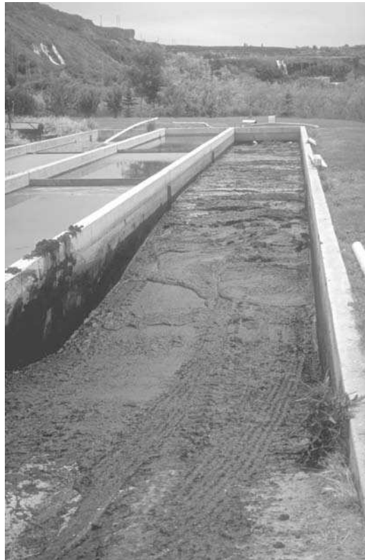
Fig. 9.8. The water in this concrete settling basin has been decanted to allow removal of the accumulated solids.
