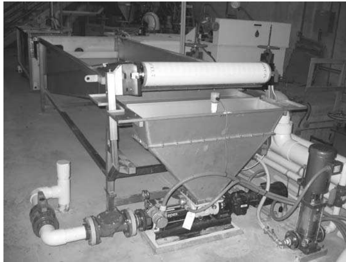
Fig. 10.11. A belt filter will scrape thickened biosolids into a collection hopper (shown centered on the drawing). The scraped biosolids are then directed to a progressive cavity pump (shown below the collection hopper) that will move the scraped biosolids to a nearby storage tank (not shown), as installed at the United States Department of Agriculture, Agricultural Research Service, National Cold Water Marine Aquaculture Center in Franklin, Maine.
