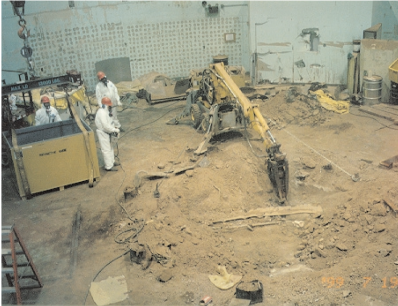
FIGURE 3.2 The BROKK demolition machine, equipped with a robotic arm, is an example of state-of-the-art technology that might be used to retrieve buried waste from Pit 9 at INEEL. Source: INEEL.
