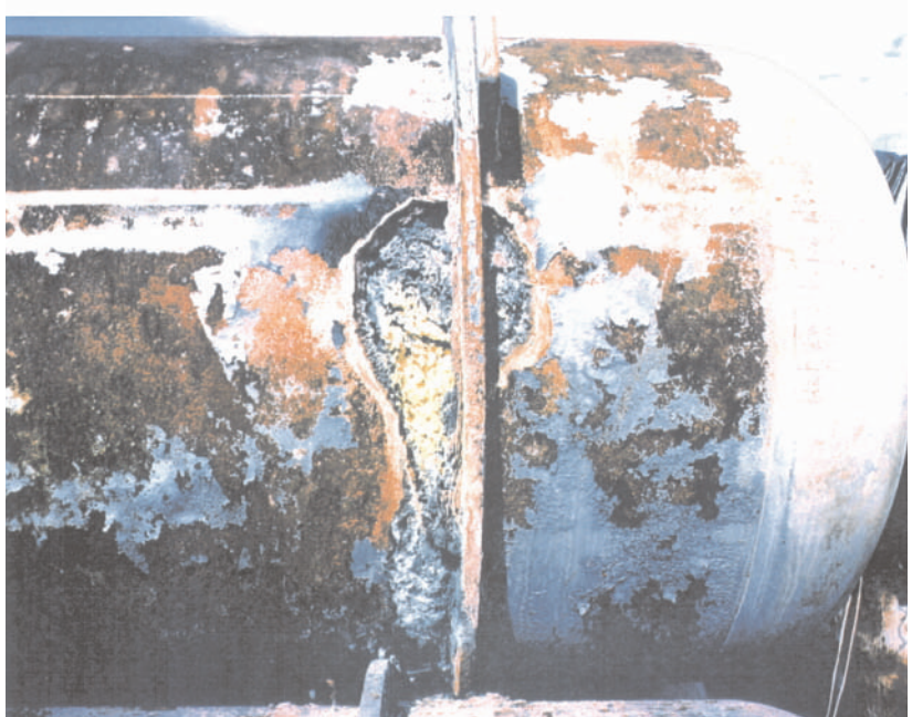
Figure 6.3 Corrosion has breached the walls of some cylinders. Breaches have tended to be self-sealing. They are repaired by welding a patch over the opening.
