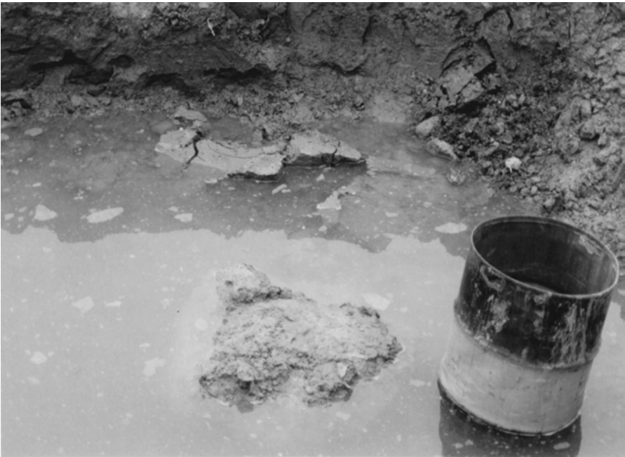
Figure 7.7 Shaft damaged by site equipment and inadequate excavation
