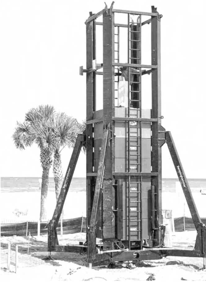
Figure 6.12 Typical Statnamic set-up for a medium-sized shaft. Reproduced by permission of Applied Foundation Testing, Inc., Florida, USA
