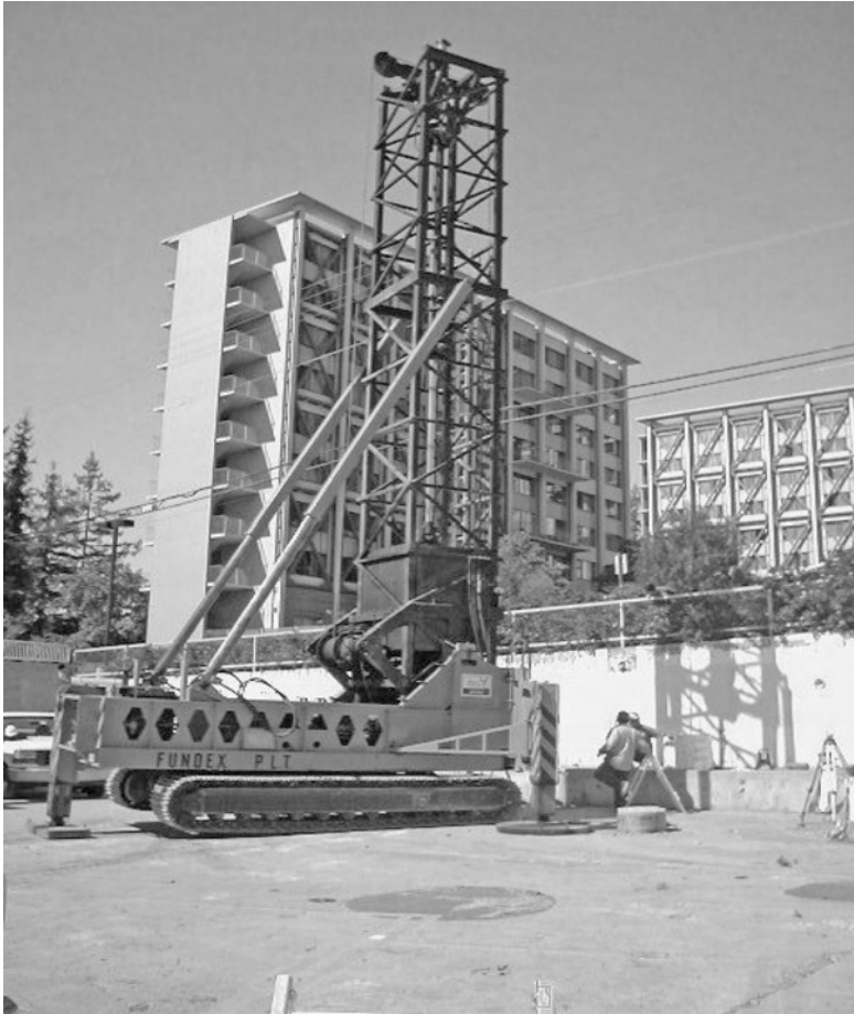
Figure 6.18 The Fundex pile-load test (PLT) rig. Reproduced by permission of American Piledriving, Inc., California, USA
