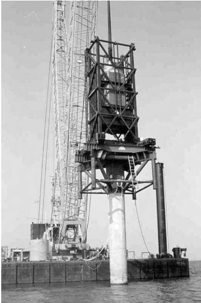
Figure 6.17 Statnamic test over water. Reproduced by permission of Applied Foundation Testing, Inc., Florida, USA
