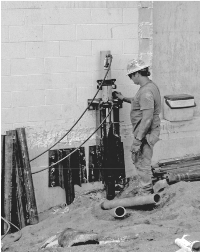
Figure 2.10 Jacking-in a steel tube micropile for structural underpinning. Reproduced by permission of Thatcher Engineering, Illinois, USA
