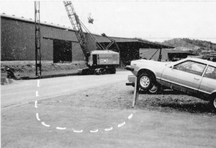
Figure 4.2 ‘You can never be sure where the end of a steel pile is going!’. Reproduced by permission of Bengt Fellenius Consultants, Alberta, Canada
