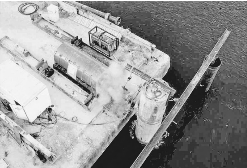
Figure 6.16 Lateral Statnamic test on a large-diameter shaft using a barge. Reproduced by permission of Applied Foundation Testing, Inc., Florida, USA
