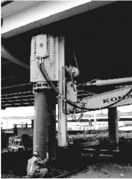
Figure 2.3 Low-profile hydraulic hammer driving under low headroom. Reproduced by permission of American Piledriving Equipment, Washington, USA
