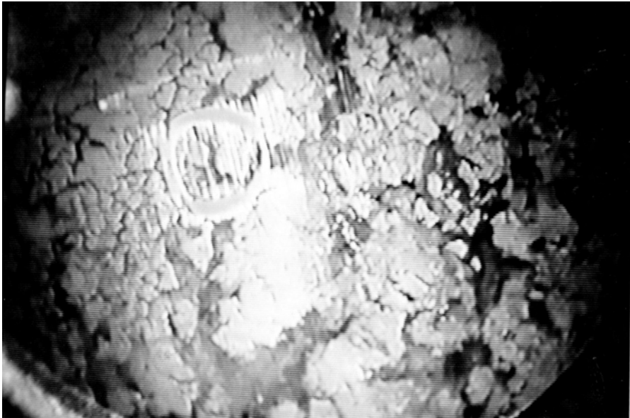
Figure 13.10 Lateral view of 'honeycomb' or leached concrete. Reproduced by permission of Stress Engineering, Inc., Texas, USA
