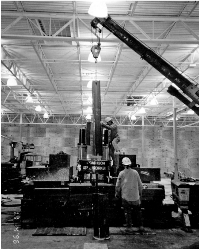
Figure 2.5 Stillworker press-in piling system used inside a building – note the steel weights stacked around the machine to increase reaction mass. Reproduced by permission of Thatcher Engineering, Illinois, USA
