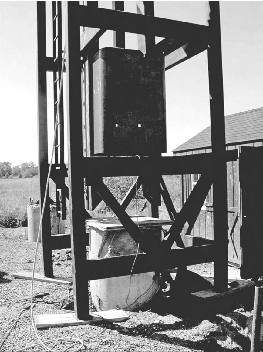
Figure 6.11 Typical 'Newton's Apple' set-up for a medium-sized shaft. Reproduced by permission of GRL Engineers, Inc., Ohio, USA
