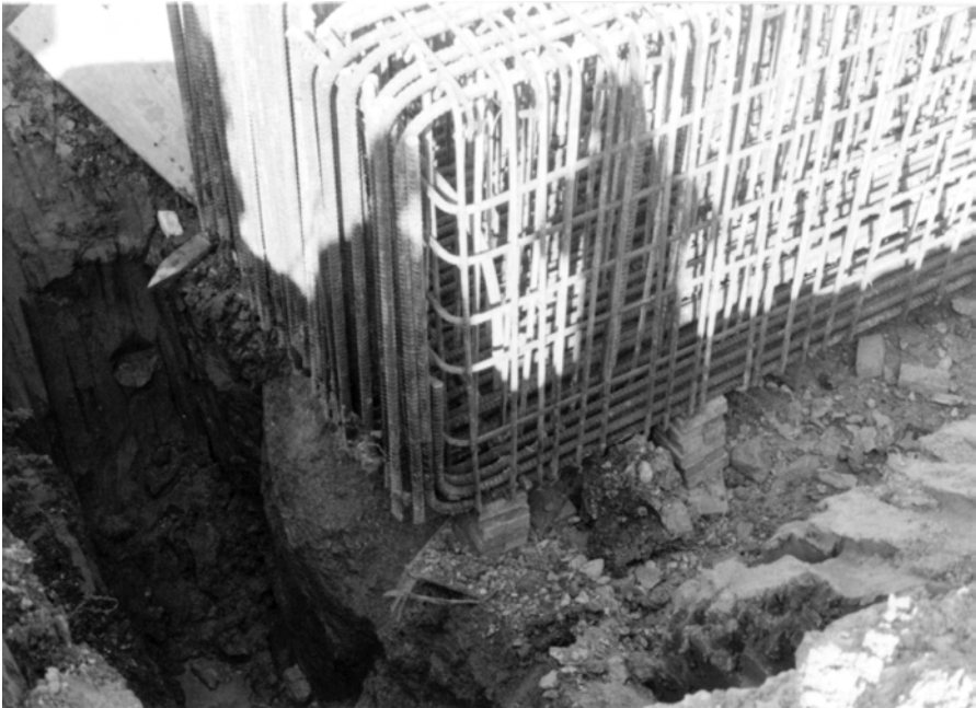
Figure 7.5 Shaft head inaccessible for testing due to a cap-reinforcing cage
