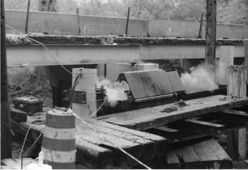
Figure 6.15 Lateral Statnamic test on a small-diameter shaft using skids. Reproduced by permission of Applied Foundation Testing, Inc., Florida, USA
