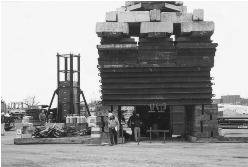
Figure 6.14 Comparison of Statnamic and a traditional kentledge for the same-sized shafts. Reproduced by permission of Applied Foundation Testing, Inc., Florida, USA
