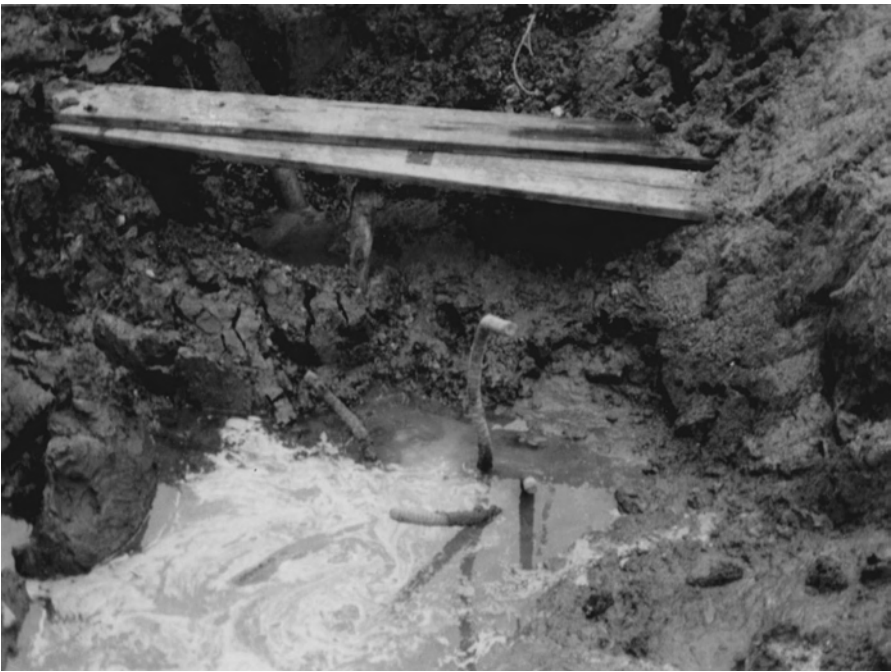
Figure 7.6 Shaft head inaccessible for testing due to inadequate excavation
