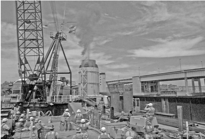
Figure 6.13 Typical Statnamic set-up for a large-diameter shaft. Reproduced by permission of Applied Foundation Testing, Inc., Florida, USA
