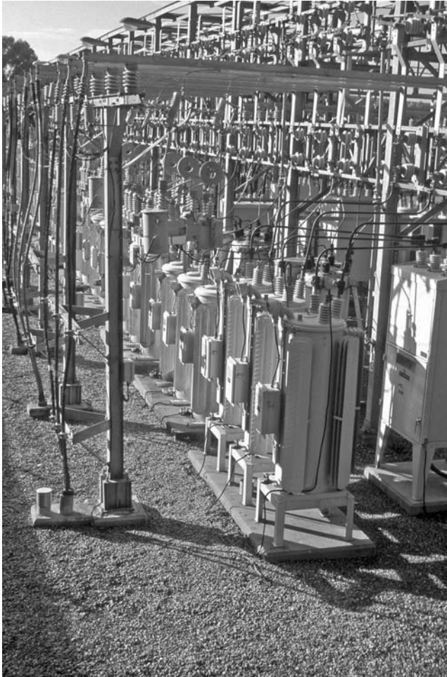
FIGURE 6.15 Aggregate surfacing in an electric substation.
