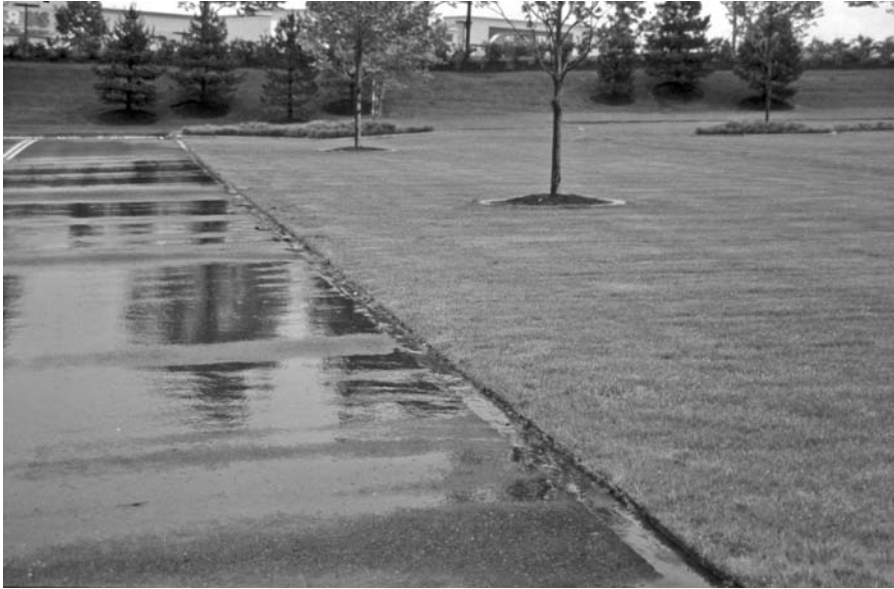
FIGURE 8.10 Drainage from the Westfarms Mall Grasspave 2 area several hours after the end of a substantial rain in May 2002.
