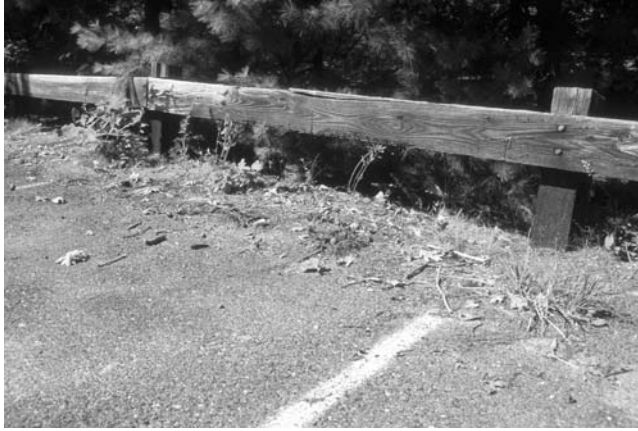
FIGURE 3.28 Timber bumper fence at the porous asphalt parking lot at Walden Pond State Reservation in Concord, Massachusetts.
