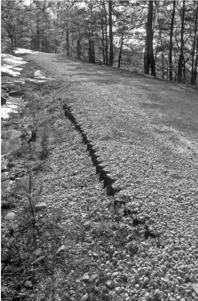
FIGURE 8.25 Aggregate maintenance road stabilized with Geoweb at Stone Mountain State Park, Georgia.
