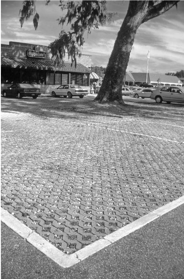
FIGURE 1.18 Open-celled concrete grids filled with porous aggregate preserving live-oak tree roots at a restaurant in Savannah, Georgia.
