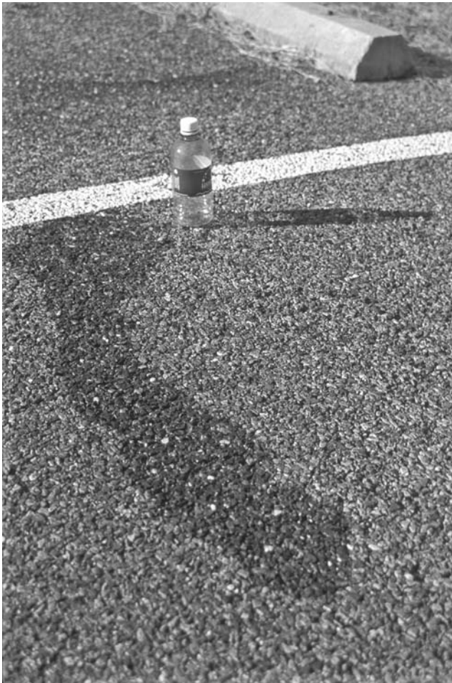
FIGURE 12.16 Partial surface infiltration in a ten-year-old porous asphalt parking lot at Quiet Waters Park, Annapolis, Maryland, in 2000.
