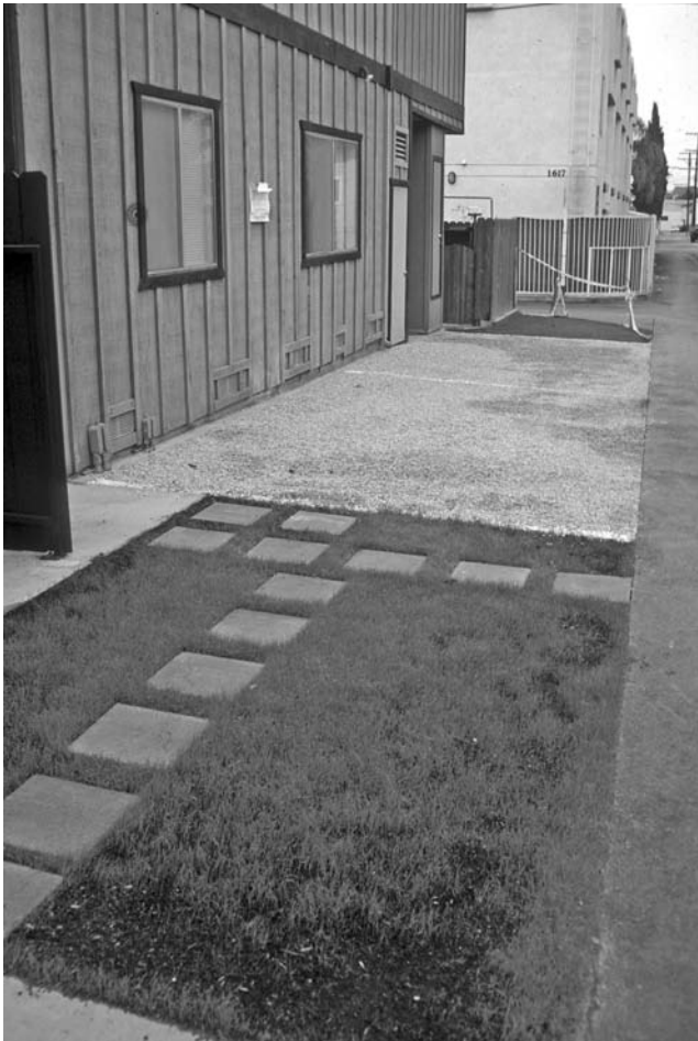
FIGURE 8.17 Residential parking spaces of Grassy Paver with aggregate fill in Santa Monica, California, soon after construction.
