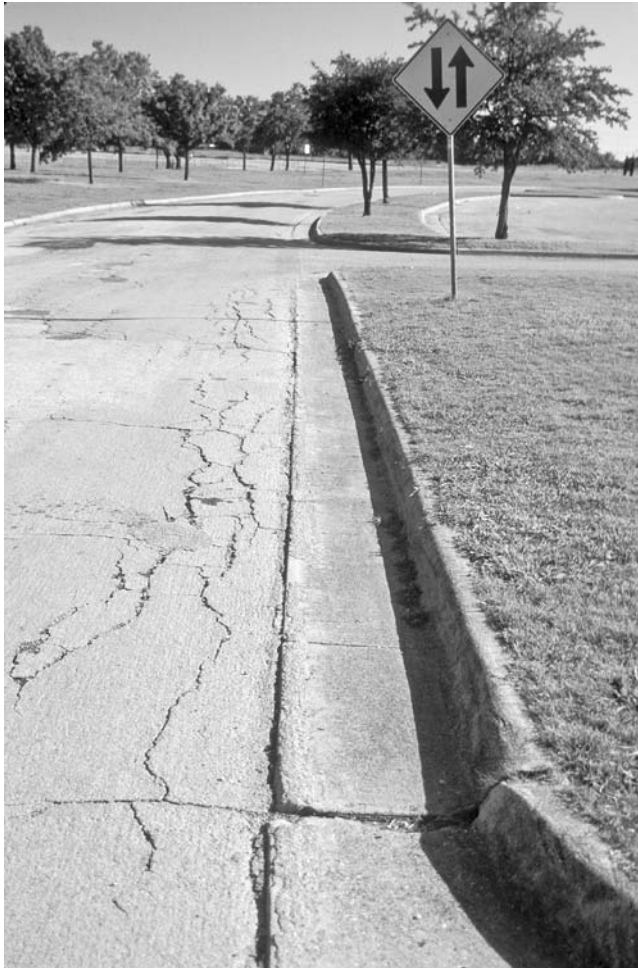
FIGURE 3.21 Cracking of a concrete curb and dense asphalt pavement resulting from swelling of the Houston black clay in Arlington, Texas.
