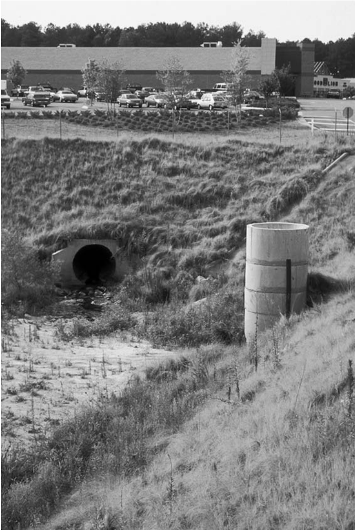
FIGURE 1.8 Detention basin in the corner of a commercial site.
