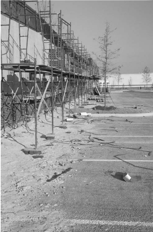
FIGURE 2.25 Construction sand spilled onto a porous concrete parking lot during erection of an adjacent wall.
