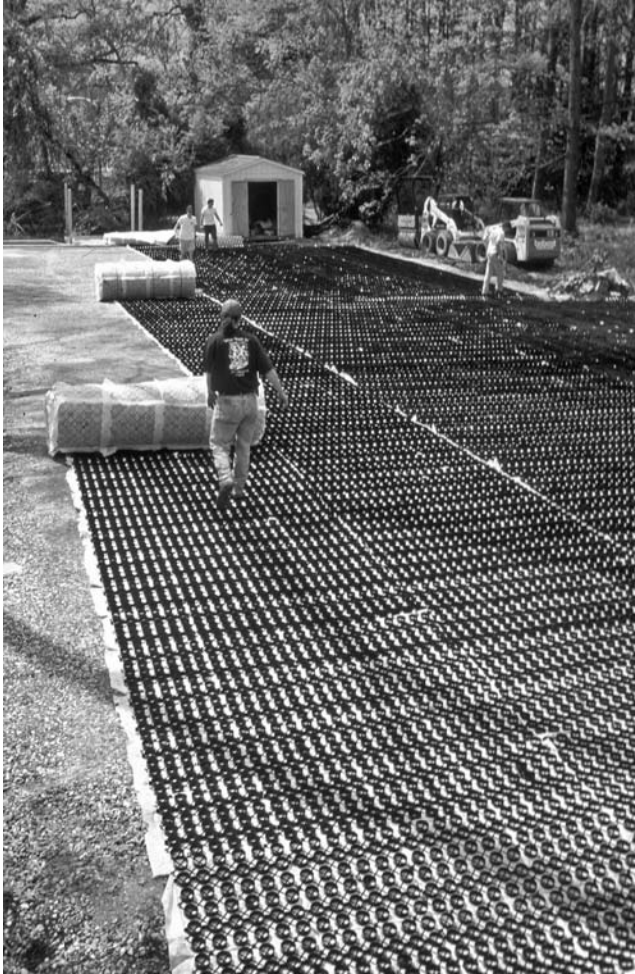
FIGURE 1.19 Plastic geocell being installed to reinforce a porous aggregate parking lot at an office building in Athens, Georgia.
