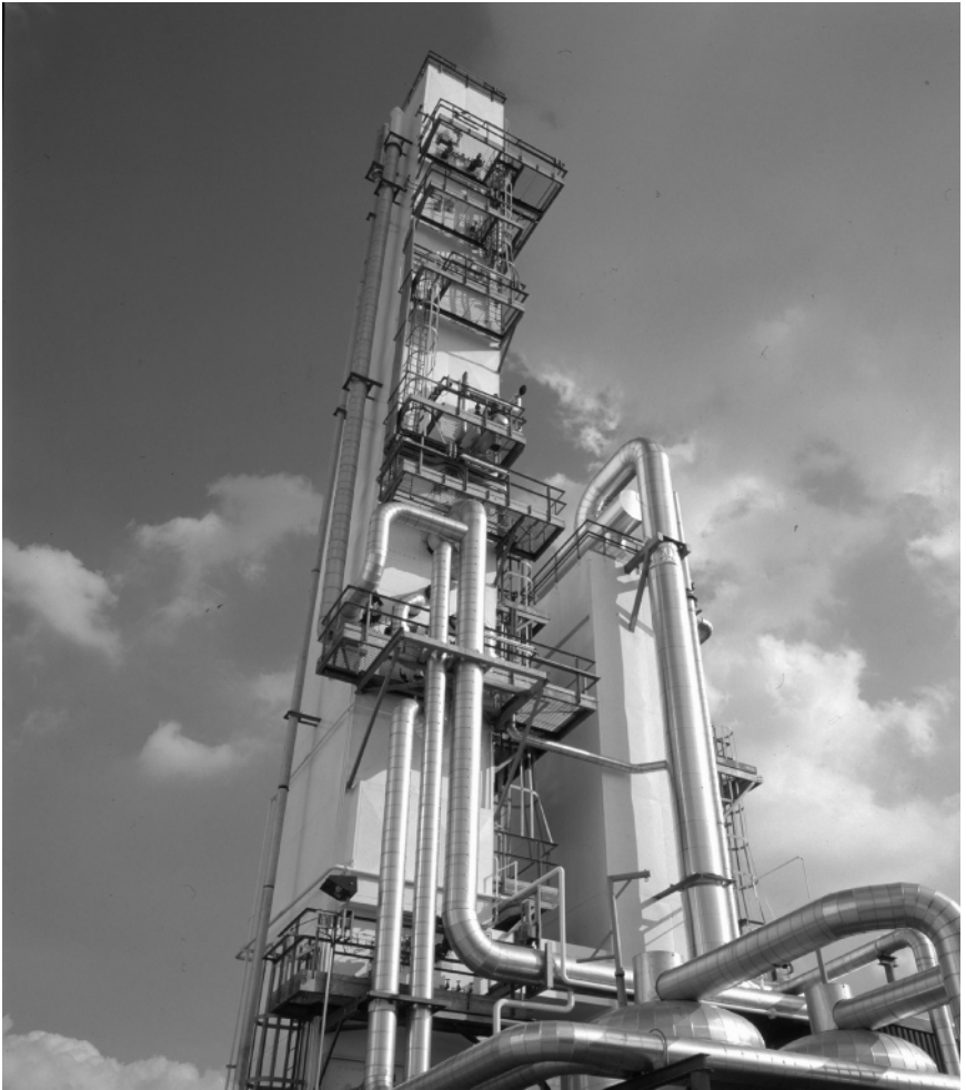
Fig. 9.5 Cryogenic liquids are only economic to manufacture on a large scale. This plant at Didcot, UK, is owned and operated by Air Products. One of the largest plants of its kind in Europe, it produces 425 t/d of liquid nitrogen as well as 175 t/d of liquid oxygen.
