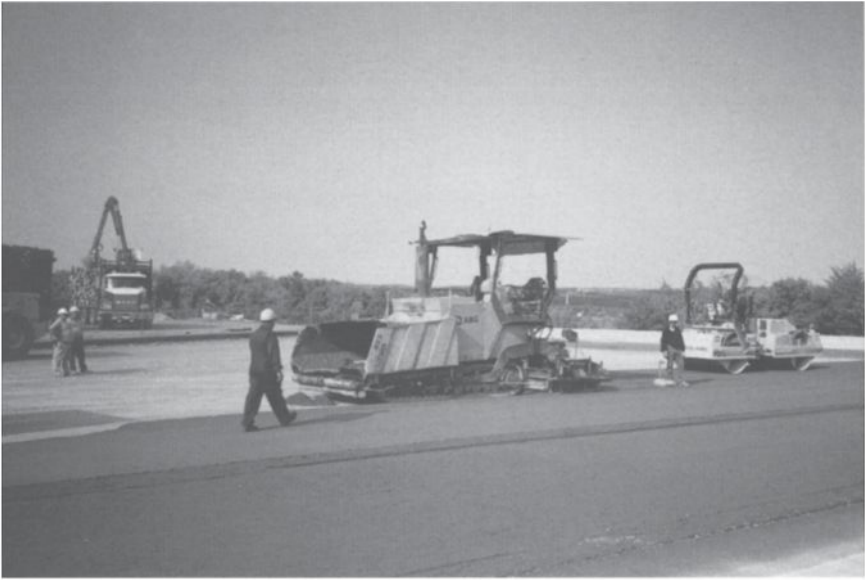
Fig. 18.13 Compacting the concrete surface and checking the unit mass with a nucleodensimeter.
