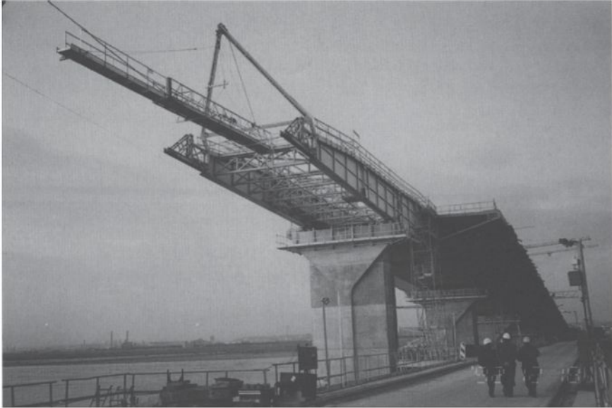
Fig. 4.16 The 605 m-long north approach built as an incrementally launched structure. The final weight of the approach was 26000 tonnes. Courtesy of Paul Acker.
