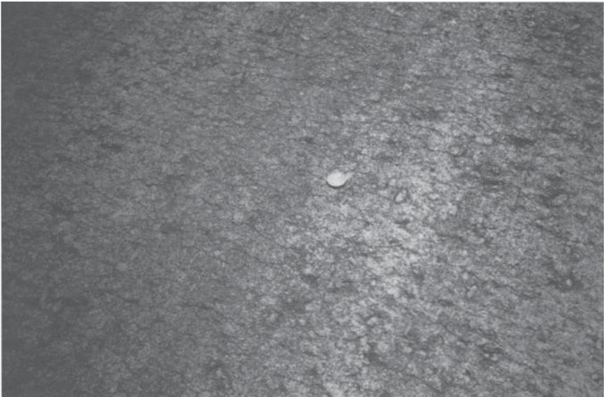
Fig. 18.14 Aspect of the concrete surface after the compaction by the vibrating rollers.
