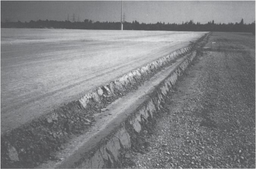
Fig. 18.9 Aspect of two 150 mm layers after their compaction. Note that the longitudinal joints of the two layers are slightly apart from each other.
