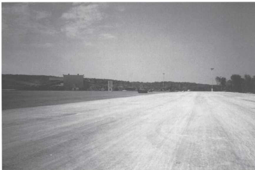
Fig. 18.15 General aspect of the finished surface, the white colour results from the use of a curing membrane.
