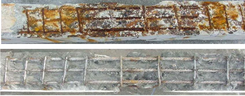
Fig. 8. Corrosion status of steel in OPCC-2 beam (Top) and FGC-3 beam (bottom)
