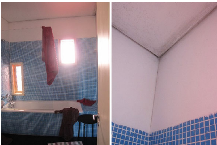
Fig. 8 Superficial Condensation in the roof of the toilet room on floor 2
