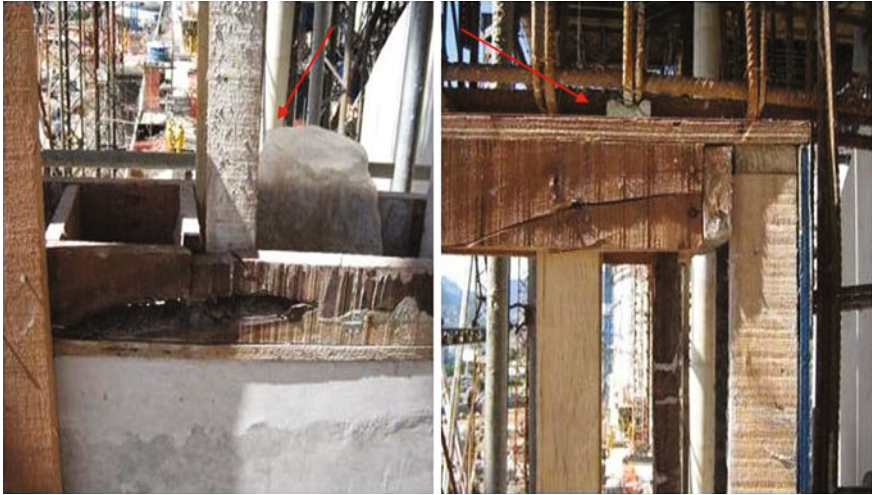
Fig. 3 Poor quality frames for exposed concrete
