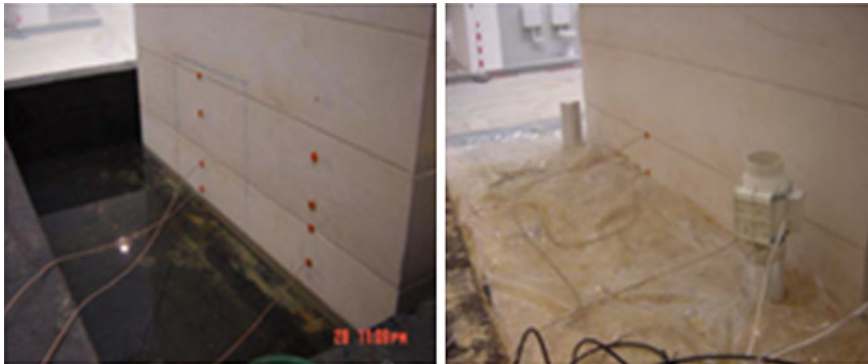
Fig. 5 Configuration 1 and 4 for experimental validation. In all configurations the wall base was immersed to a height of 8 cm to simulate rising damp. Additionally, the moisture front was monitored by probes at various points in the wall. Configurations without and with a ventilation system are presented (Torres 2004)
