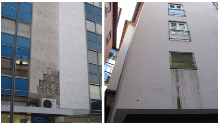
Fig. 1 State of degradation that implies the adoption of late corrective measures
