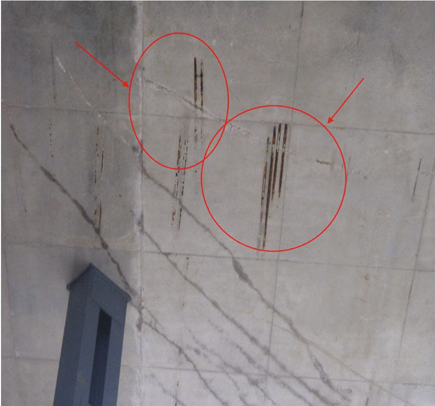
Fig. 4 Concrete reinforcement exposed
