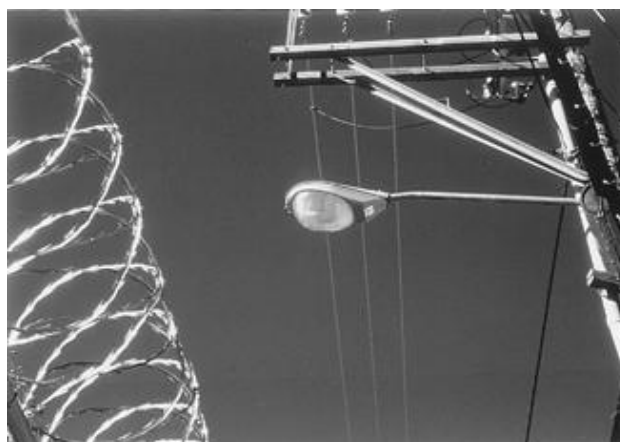
Figure 29-20. Use of a pole-mounted luminaire to light fenced perimeter areas.
