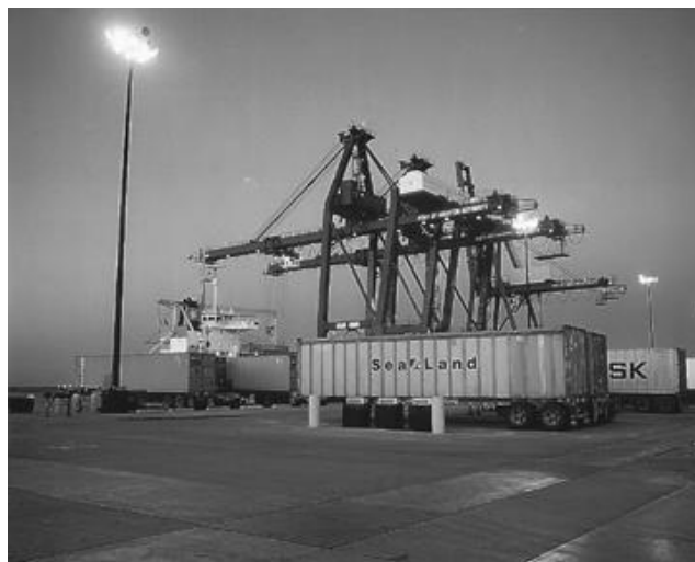
Figure 19-33. High-mast floodlights located to illuminate the dock area while reducing glare for the crane operators and cargo handlers.
