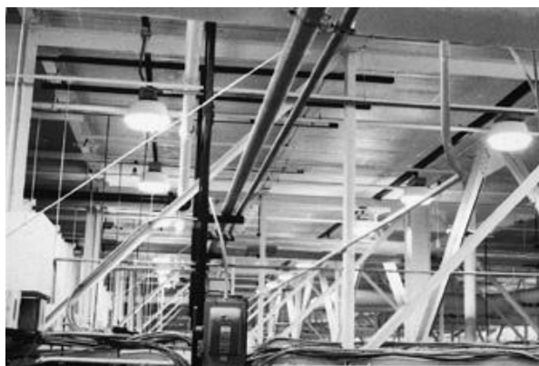
Figure 19-2. High-reflectance finish on structural elements increases the luminance surrounding the luminaires and reduces the effect of the luminaire as a "glare" source.
