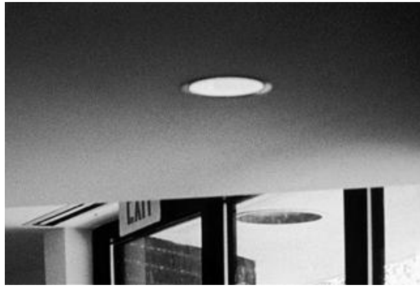
Figure 29-14. A ceiling soffit can block the line of sight to an exit sign.
