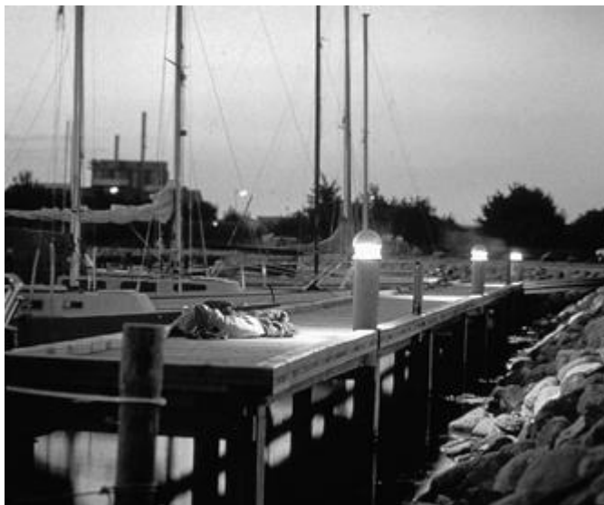
Figure 21-11. Bollard luminaires illuminate the immediate surroundings in a docking area.
