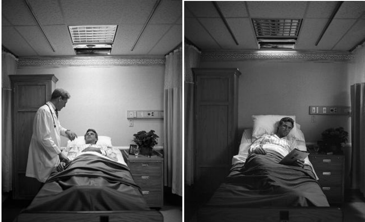
Figure 16-1. Patient room lighting. Left, examination light, which can be controlled with a wall switch by hospital staff, utilizes compact fluorescent lamps for excellent color rendition. Right, reading lighting, which positions light directly onto the patient's reading material with no reflected glare.
