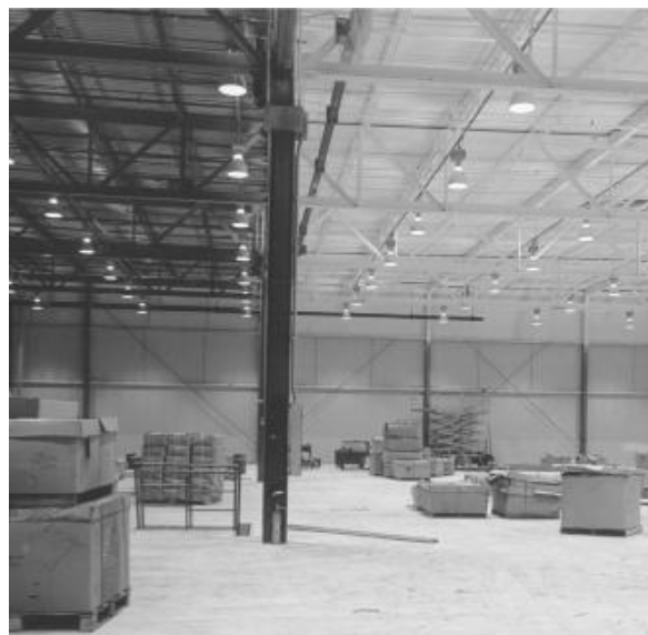
Figure 19-8. The importance of a white ceiling in an industrial facility is shown in this plant under construction. Note the improved visual environment in the right bay (where the painters have finished the ceiling) compared to that in the left (as yet, unpainted). The illuminance in the right is substantially higher, too.
