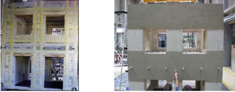
FIGURE 2. Prototypes repaired with GFRP laminates (right) and GFRP grid bonded with cementitious mortar (left)
