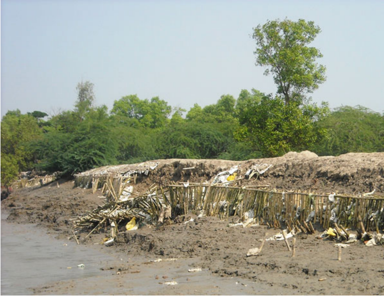
Fig. 2.6 Earthen embankment typical of Sunderbans noted with basal destruction
