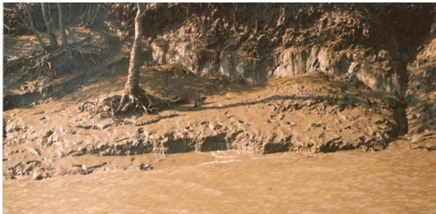
Fig. 7.2 River bank erosion through sagging-down of bank materials
