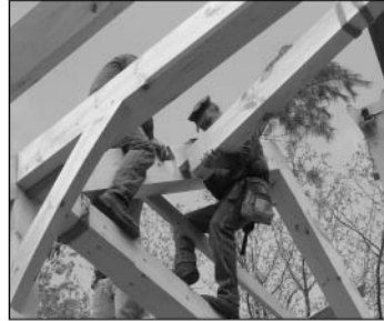
Figure 3.5-8. Timber framing has experienced a revival in popularity. (Photo by DeStefano & Chamberlain, used with permission)
