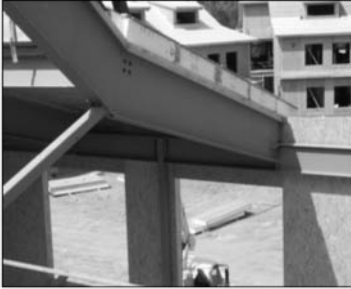
Figure 3.5-7. SIP roof and wall cladding over structural steel on a school in Cherokee, N.C. (Photo by Panelwrights, used with permission)
