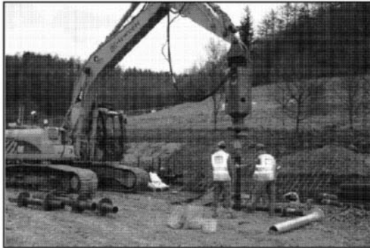
Figure 5.3-3. Piles being installed at the Dalby Forest Visitors' Center (Photo courtesy Miller Construction)
