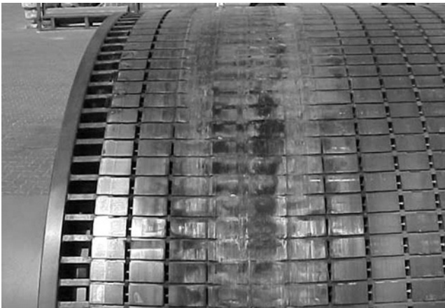
Figure 10.8 3-Phase, 4350 HP/3245 kW, 11 kV, 204 A, 50 Hz, 592 r/min, p.f. = 0.88, efficiency = 95% SCIM. Catastrophic rotor-to-stator rub and stator winding failure in a brand new SCIM, August 2004. A segmental laminated rotor core—radial movement of the rotor core.
