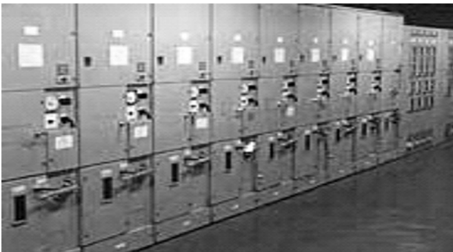
Figure 4.7 Typical layout of HV circuit breakers and instrumentation cubicles for HV motors.
