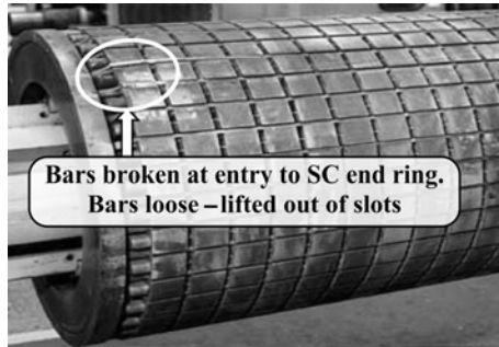
Figure 3.19 Fabricated copper cage winding with two broken bars, which have lifted out of the slots, caused by too many sequential DOL starts, bars were not originally tight enough in the slots. Source: Thomson and Fenger [3.18]. Reproduced with permission of IEEE.
