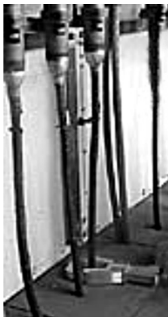
Figure 4.9 MESA clip-on CT around one of the 3-phases external to the motor's circuit breaker in a power station.
