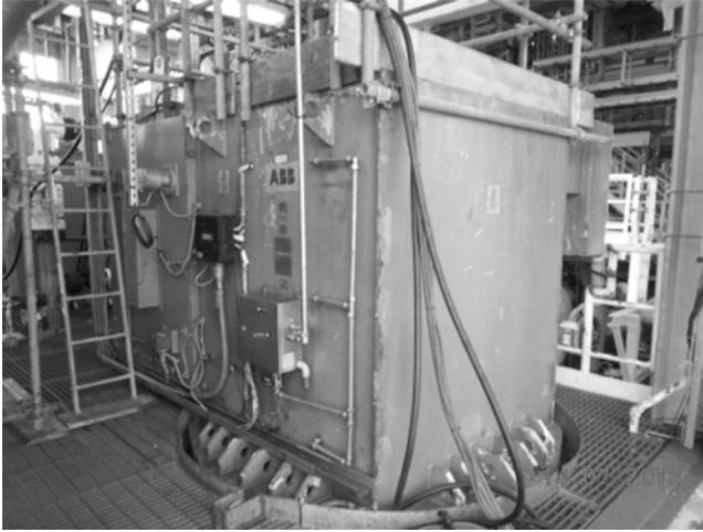
Figure 11.38 Motor being MCSA tested.
