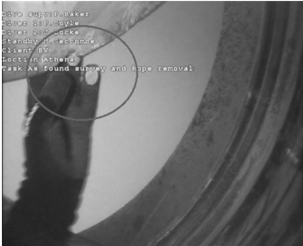
Figure 8.47 Chip on propeller blade. Reproduced with permission of BW Offshore (UK) Ltd., Aberdeen, Scotland.
