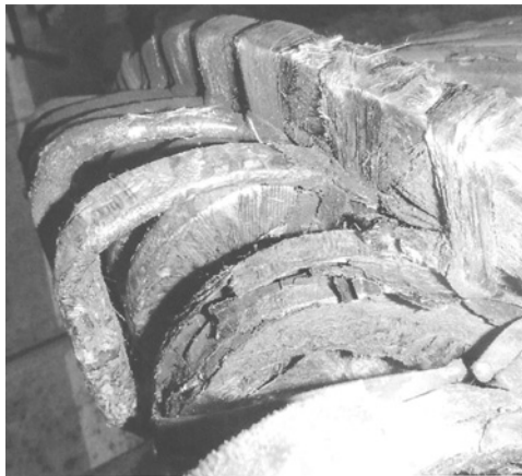
Figure 12.4 Example of failure due to shorted turns in a 6.6 kV SCIM.
