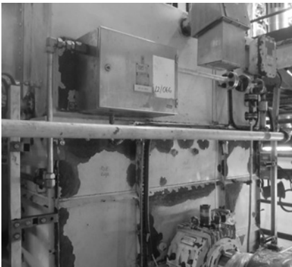
Figure 6.23 View of DE of the motor. Reproduced with permission of Quartzelec, Aberdeen, Scotland.
