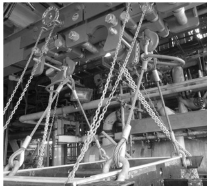
Figure 6.26 Photo of the crane set up. Reproduced with permission of Quartzelec, Aberdeen, Scotland.
