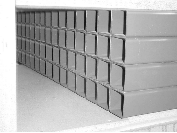
Fig. 9.20. Photograph of a duct wall lined with resonators which are realized by rigidly terminated pipes of depth d
