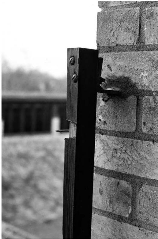
Figure 15.12 The crack path in a failed end post.
