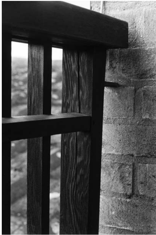
Figure 15.11 An 18-inch crack in another balustrade.
