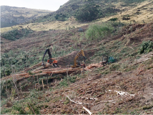
Figure 5. Feller, buncher, and log forwarder at Charteris Bay, near Christchurch, New Zealand
