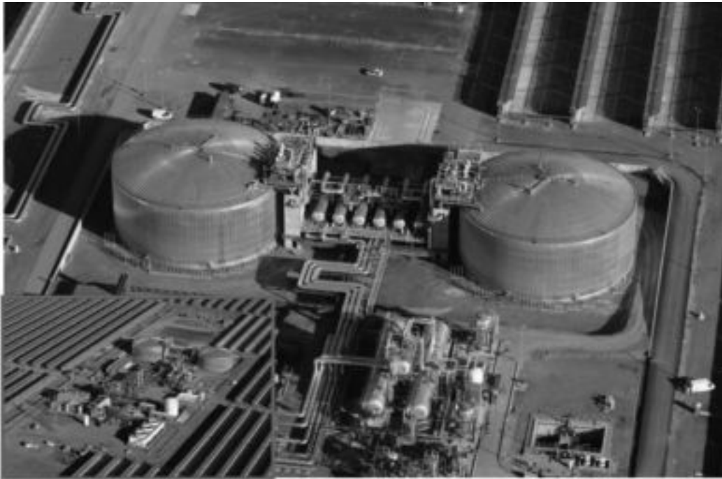
FIG. 3.11 AERIAL VIEW OF POWER ISLAND AND DETAIL OF MOLTEN-SALT STORAGE TANKS AND HEAT EXCHANGERS OF ANDASOL PLANT. THIS 50 MW PLANT STORES THERMAL ENERGY EXCESS IN 28,500 TONNES OF NITRATE MOLTEN SALTS ABLE TO PROVIDE UP TO 7.7 EQUIVALENT HOURS OF OPERATION AT NOMINAL CAPACITY (ANDASOL-I PLANT, GUADIX, SPAIN) (Source: ACS/Cobra Energía (Spain))
