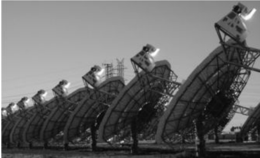
FIG. 3.18 ROW OF DISH-STIRLING SYSTEMS (STIRLING ENERGY SYSTEMS SUNCATCHER) OF 25 KW EACH AT THE MARICOPA SOLAR PLANT IN ARIZONA (Source: Stirling Energy Systems)
