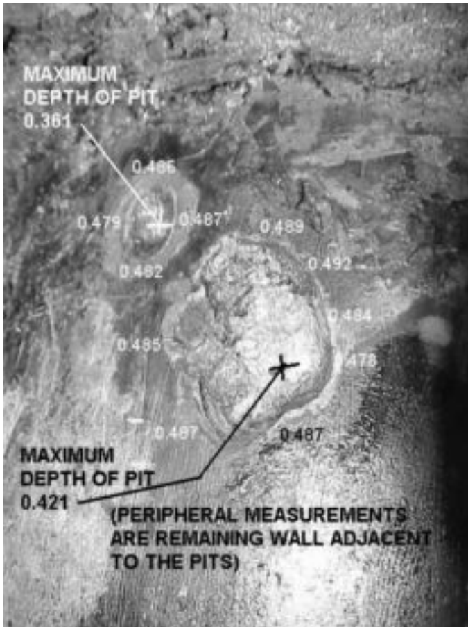
FIG. 22.5 EXAMPLE OF LOCALIZED WALL THICKNESS LOSS DUE TO MICROBIOLOGICALLY INFLUENCED CORROSION (MIC) [18]
