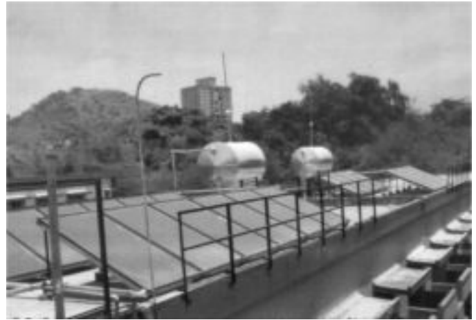
FIG. 4.13 SOLAR WATER HEATING SYSTEM AT IIT BOMBAY, MUMBAI [23]
