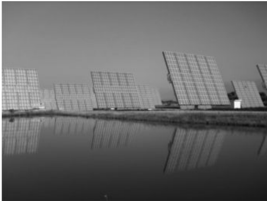
FIG. 1.11 AN ARRAY OF 25-KW AMONIX DESIGNS IN SPAIN AT THE GUASCOR FOTON INSTALLATION LICENSE PARTNER OF AMONIX. NEWER UNITS HAVE MUCH HIGHER POWER OUTPUT BECAUSE OF THE USE OF MULTIJUNCTION CELLS (From AMONIX)
