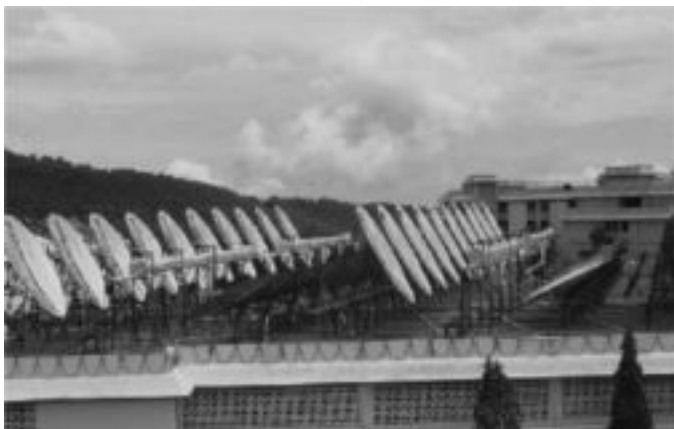
FIG. 4.12 SOLAR COOKING SYSTEM AT TIRUMALA TIRUPATI DEVASTHANAM, ANDHRA PRADESH [20]
