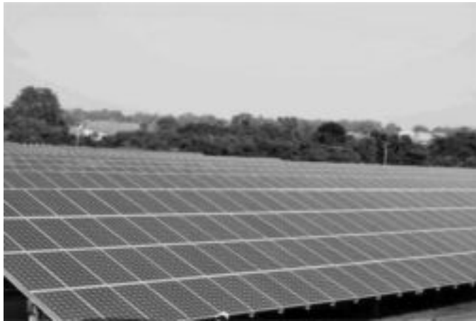
FIG. 4.7 1 MW SPV POWER PLANT INSTALLED BY WEST BENGAL GREEN DEVELOPMENT CORPORATION LIMITED AT JAMURIA VILLAGE IN ASANSOL, WEST BENGAL [9]
