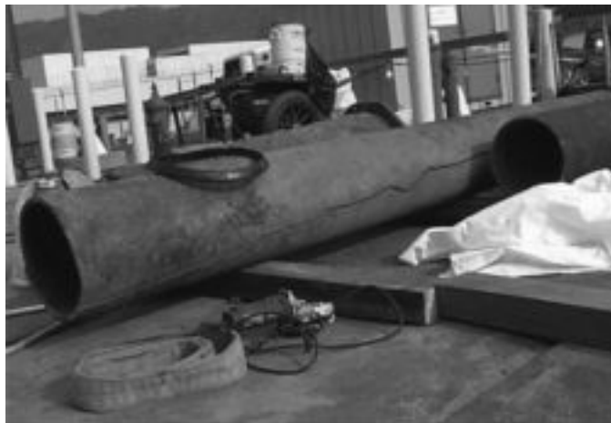
FIG. 22.4 AN EXAMPLE OF A FAILURE IN CAST IRON PIPING [18]
