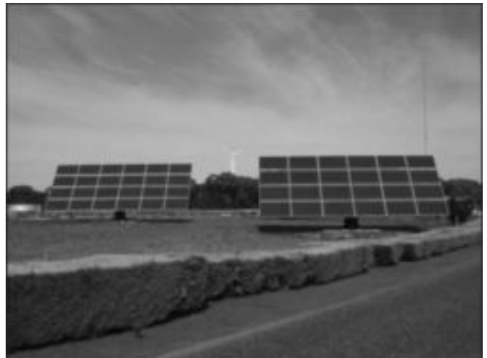
FIG. 28.9 SOLAR PV INSTALLATION, SOLON XL MOVERS (Source: Hydro Tasmania)
