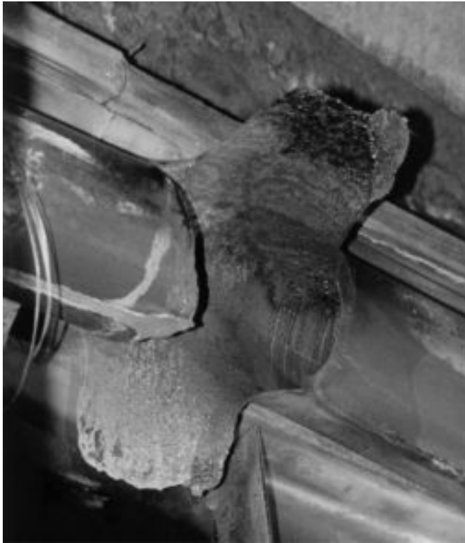
FIG. 22.1 RUPTURE OF A 6-IN. (152.4 MM) FEEDWATER PIPE IN AN AREA THINNED BY INTERNAL CORROSION [5]
