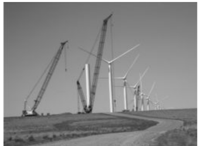
FIG. 8.17 CRANES USED TO ERECT TOWER AND ROTOR SECTIONS AT A WIND FARM NEAR BLISS, ID (Photo Courtesy of Todd Haynes, 2008)
