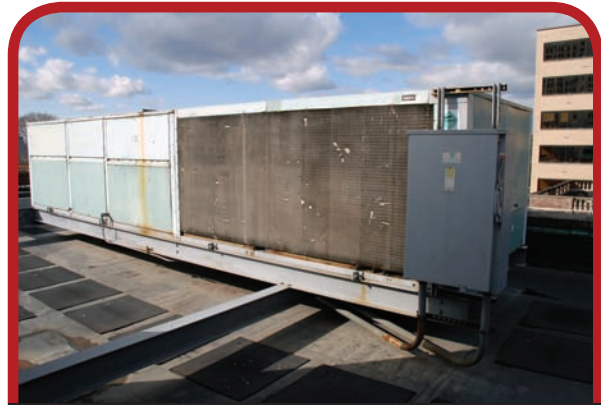
Roof top multi-zone packaged unit. (Delmar/Cengage Learning) FIGURE 17.17
