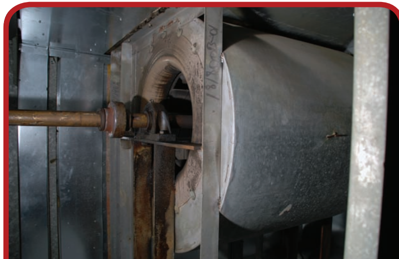
Commercial and industrial blower unit. (Delmar/Cengage Learning)
