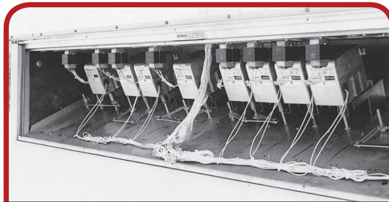
Dampers of multi-zone roof top packaged unit. (Delmar/Cengage Learning)
