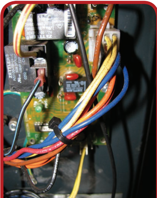
Electronic module used on a heat pump with a diagnostic function. (Delmar/Cengage Learning)
