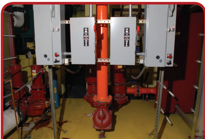
Disconnect switch installed on equipment. (Delmar/Cengage Learning) FIGURE 8.8
