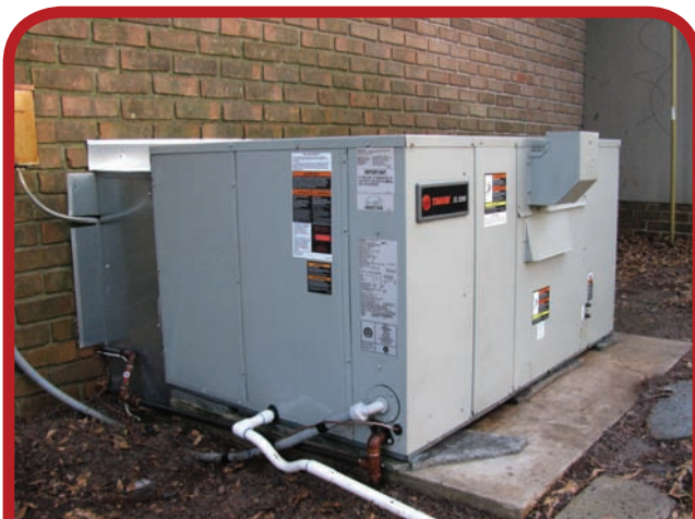
Gas heat electric air-conditioning packaged unit. FIGURE 16.27 (Delmar/Cengage Learning)
