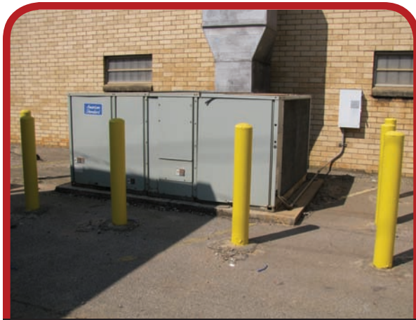
Large packaged unit showing ground level installation. FIGURE 17.16 (Delmar/Cengage Learning)
