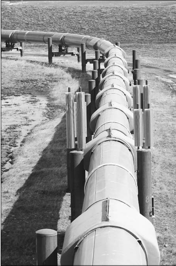
A section of the Alaska Pipeline, which carries crude oil from the state's northern slopes to Valdez on Alaska's southern coast. (PhotoDisc)
