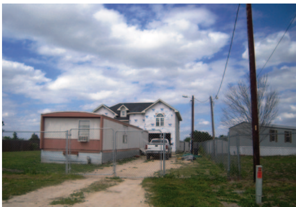
Fig. 15.9 Manufactured home (trailer in front) with custom home under construction at the rear. Redwood
