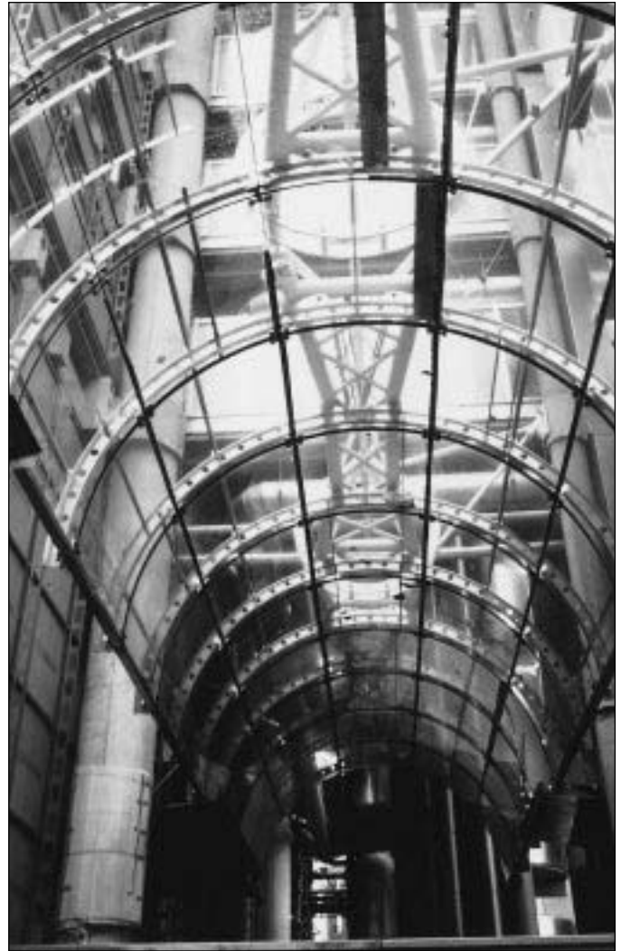
Fig. 7.5 Entrance canopy, Lloyds headquarters building, London, UK, 1986; Richard Rogers and Partners, architects; Ove Arup & Partners, structural engineers. The curved steel ribs with circular 'lightening' holes are reminiscent of structures found in the aerospace industry. (Photo: Colin McWilliam)
