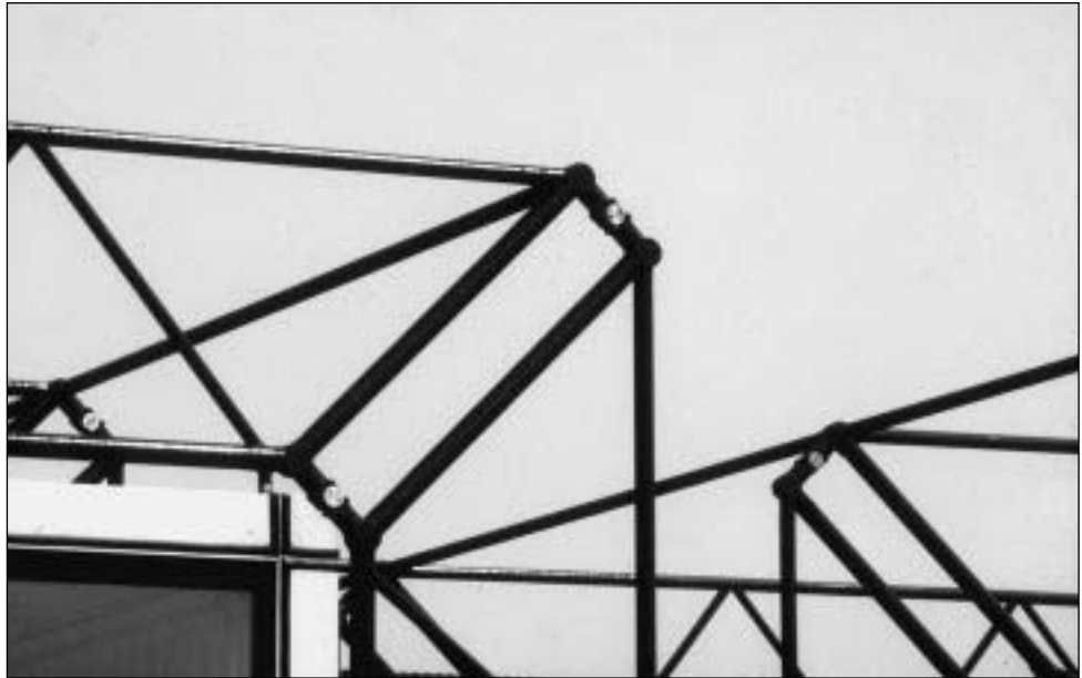
Fig. 7.28 Patera Building; Michael Hopkins, architect; Anthony Hunt Associates, structural engineers. The ingenious use of pin connections and cast nodes allowed a fully rigid joint to be made between the principal elements which could be easily assembled. (Photo: Anthony Hunt Associates)
