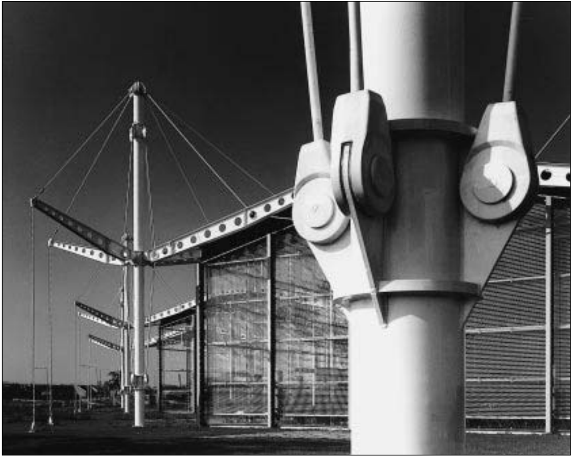
Fig. 3.19 Renault Sales Headquarters, Swindon, UK, 1983; Foster Associates, architects; Ove Arup & Partners, structural engineers. Joints in steelwork can be detailed to look very neat and to convey a feeling of great precision. (Photo: Alastair Hunter)
