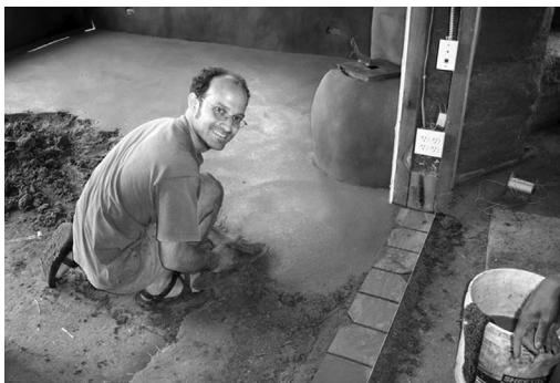
Figure 6.4 Illustration showing the method for installing an earth floor. Source: Brian “Ziggy” Liloia, “Building My Cob House” blog.
