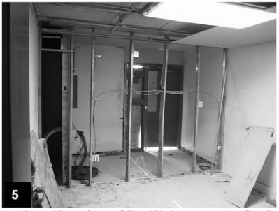
5 Interior – View of new Office Workspace on the first floor which is scheduled to be completed by third week of January 10, 2012
