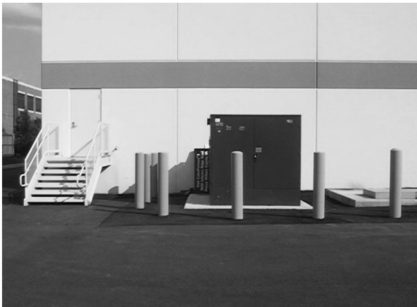
Figure 9.24 Illustration of a Transformer located outside a facility and protected by bollards.
