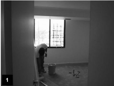
1 Interior – View of work in progress on Unit 302 on the third floor of the ABC Apartments. About 230 units are now complete and 12 others are in progress. Unit is scheduled to be completed by end of January 8, 2012
