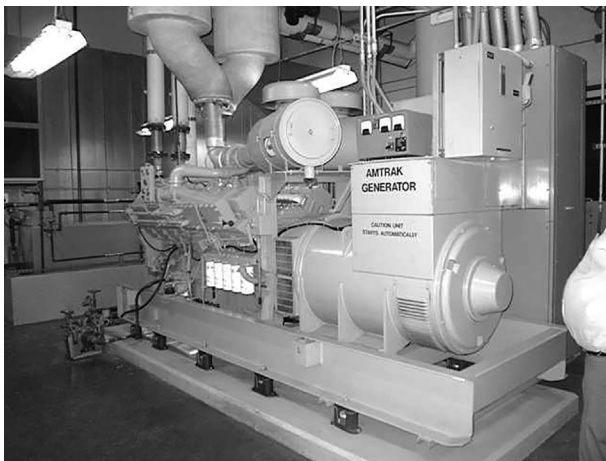
Figure 9.23 Photo of an Amtrak generator for emergency backup power inside a building.
