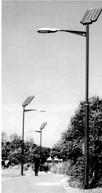
Figure 9.26 Example of solar power LED street lighting with automatic on–off, lasts for four to five nights after fully charged. Source: Hankey Asia Ltd.
