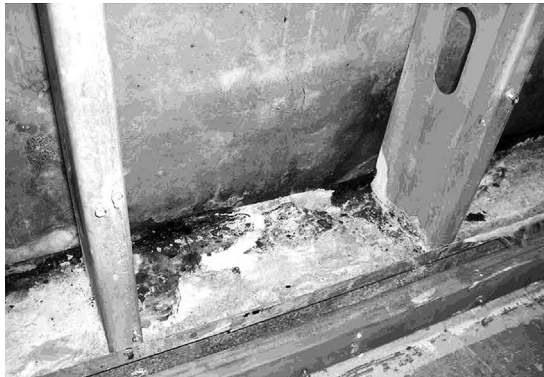
Figure 9.5 Photo showing effects of water penetration contributing to mold growth.
