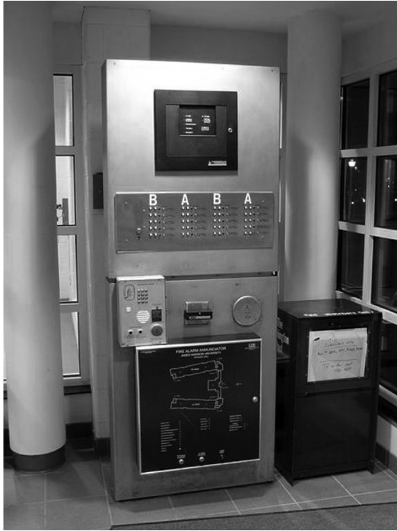
Figure 9.37 A Siemes MXL fire alarm control panel (top) and graphic annunciator (bottom) for Potomac Hall, at James Madison University. Photograph by Ben Schumin, (source: Wikipedia).
