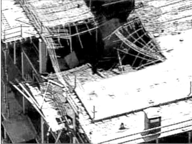
Figure 16.3a 14 people were injured when a section of the roof of the “The Landmark,” a $140 million dollar high-rise building collapsed onto the 13th and 12th floors as concrete was being poured for the building’s roof. Source: CBS Broadcasting Inc.
