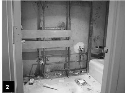
2 Interior – View showing work in progress on the upgrading of the Bathroom plumbing in Unit 1104 on the eleventh floor. Unit is scheduled to be completed by January 10, 2012
