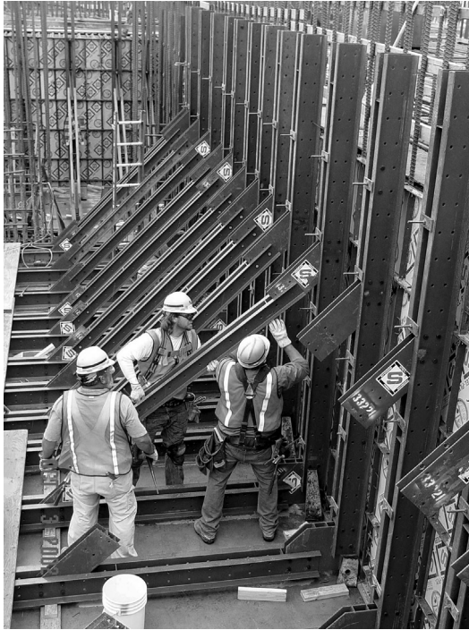
Figure 6.10 Photo of carpenters setting concrete formwork for high-level waste facility pit walls. Source: Bechtel Corporation.
