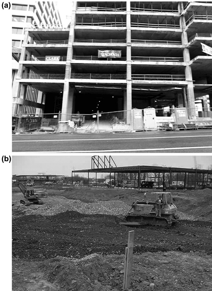
Figure 15.5 (a) An office building under construction in Arlington, Virginia. A building sign shows the name of the lending institution and the general contractor. It may be prudent to send promotional mail to the bank to have your firm's name on their contractor list and also a letter to the construction company to seek subcontracting work. (b) Construction underway in Bowie Town Center, Maryland offers opportunities for subcontracting work.
