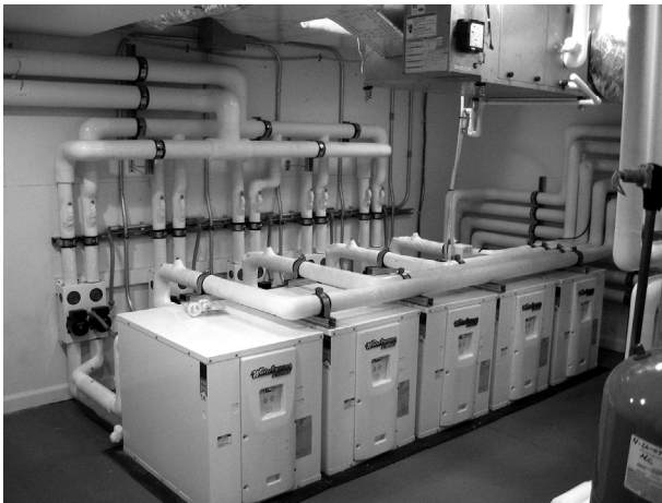
Figure 9.11 A residential geothermal heat pump system. Source: Climate Heating and Cooling, Inc.
