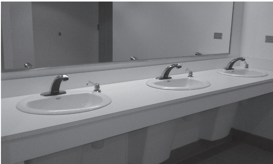
Figure 5.1 Implementing commercial bathroom lavatories with sensors help to reduce water consumption and could help to achieve WE Prerequisite 1 of the LEED CI rating system. Photo courtesy of Stephen Martorana, LEED AP BD+C
