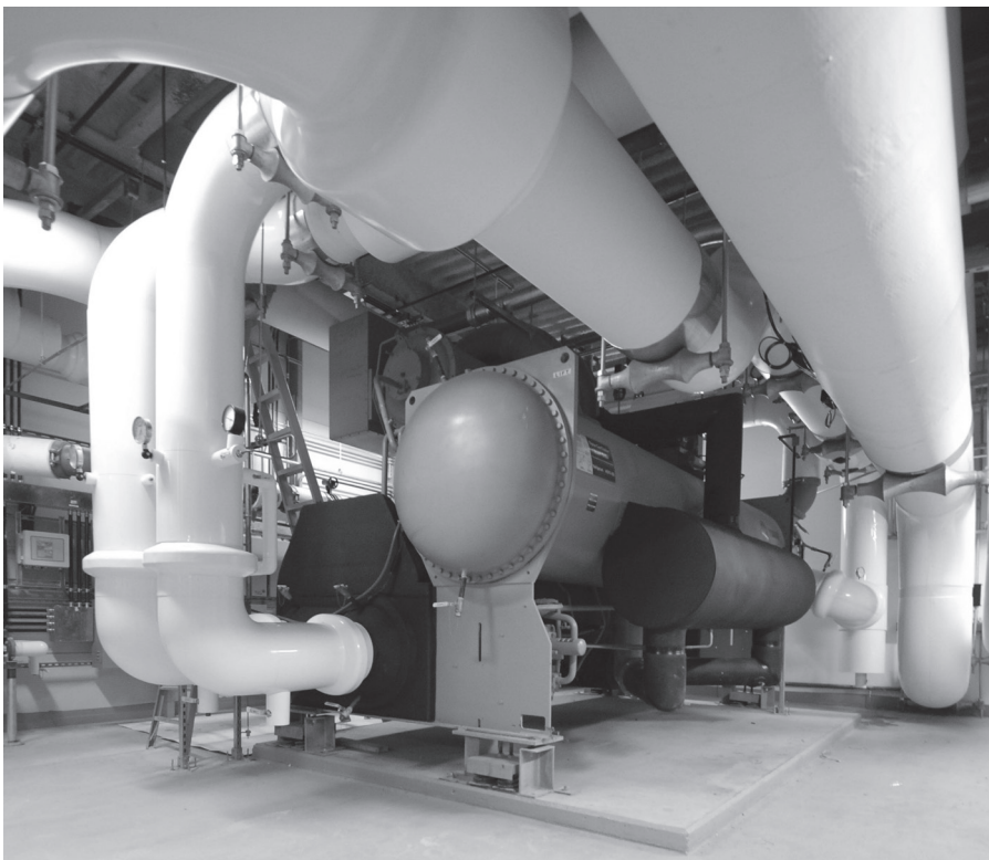
Figure 6.5 Installing high-efficiency chillers can help to achieve energy performance and savings goals.
