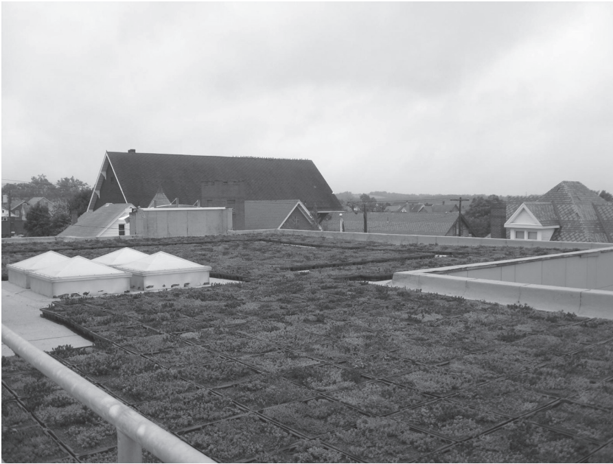
Figure 4.7 This green roof at the Allegany County Human Resources Development Commission's community center in Cumberland, Maryland, minimizes impervious areas to reduce stormwater runoff. Photo courtesy of Moshier Studio
