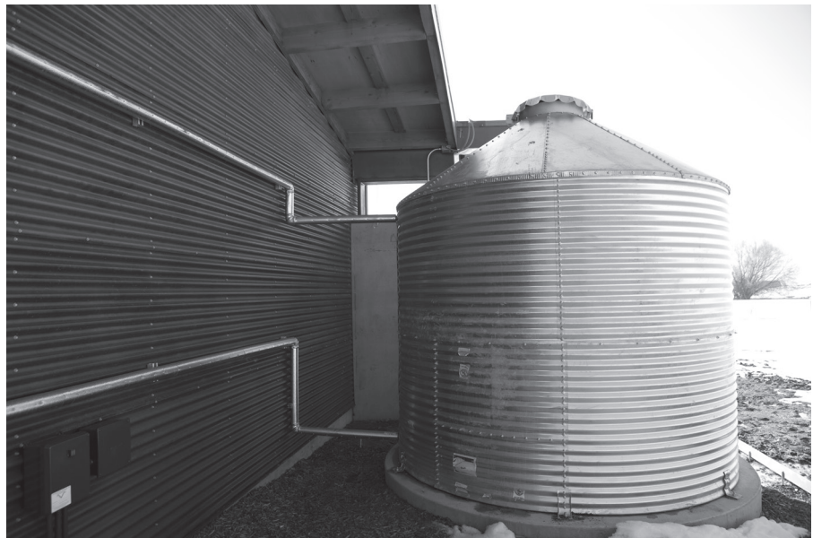
Figure 4.16 Stormwater is collected on-site and stored in cisterns at the Utah Botanical Center’s Wetland Discovery Point building and used to flush toilets, as well as irrigate the site, thus reducing the need for potable water. Photo courtesy of Gary Neuwander, Utah Agricultural Experiment Station
