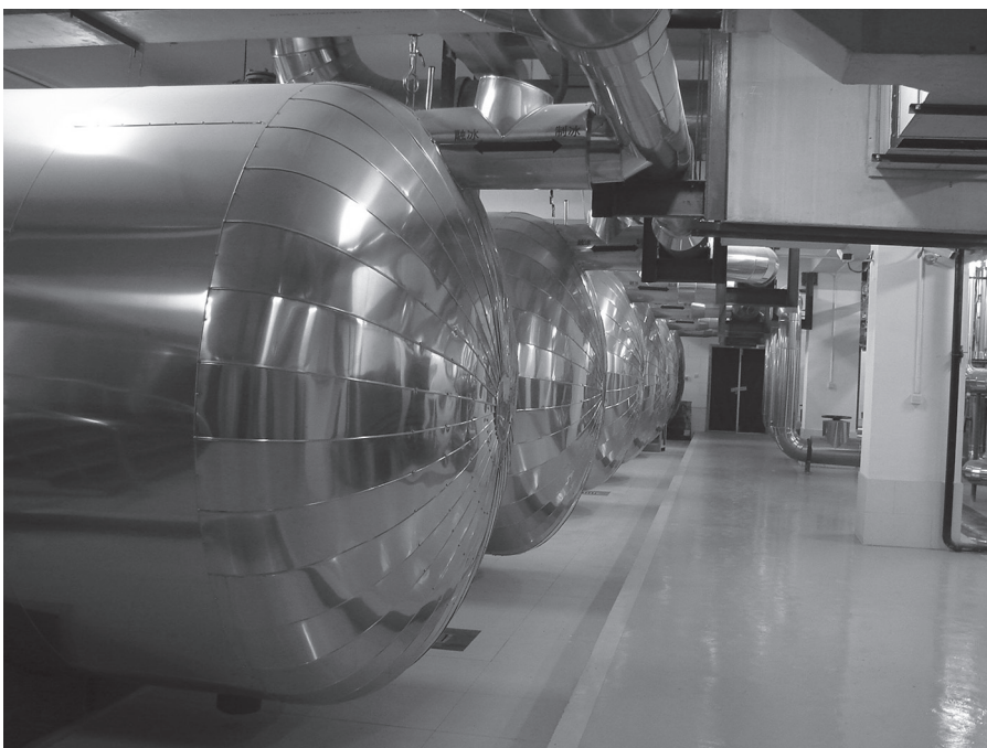
Figure 6.6 Ice ball thermal energy storage helps to provide cooling during the day from ice generated at night to reduce energy demands.
