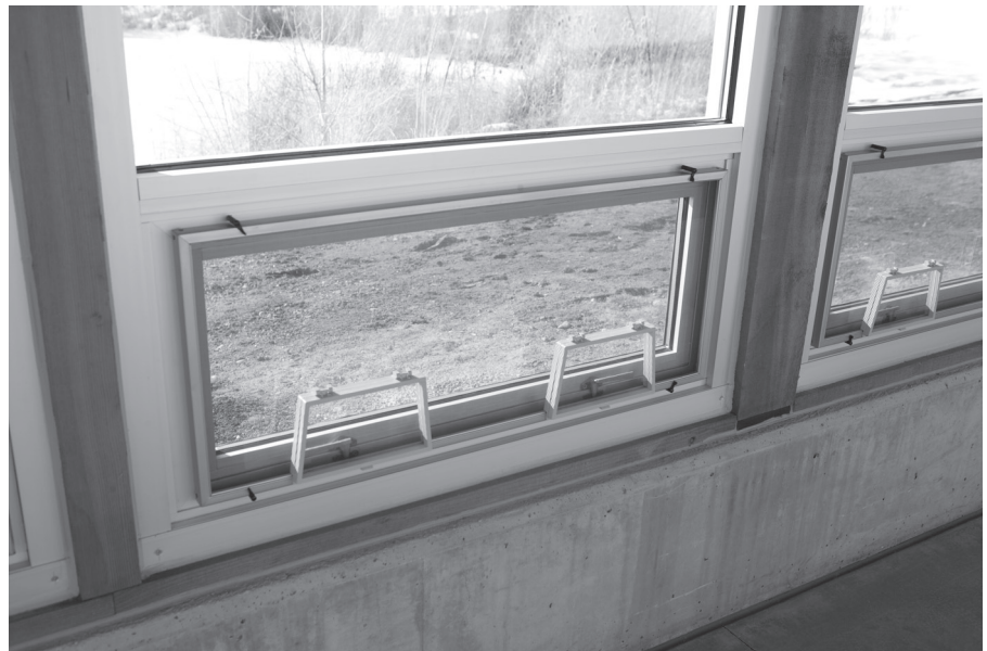
Figure 8.2 Providing operable windows offers building occupants access to means of adequate ventilation. Photo courtesy of Gary Nevenswander, Utah Agricultural Experiment Station
