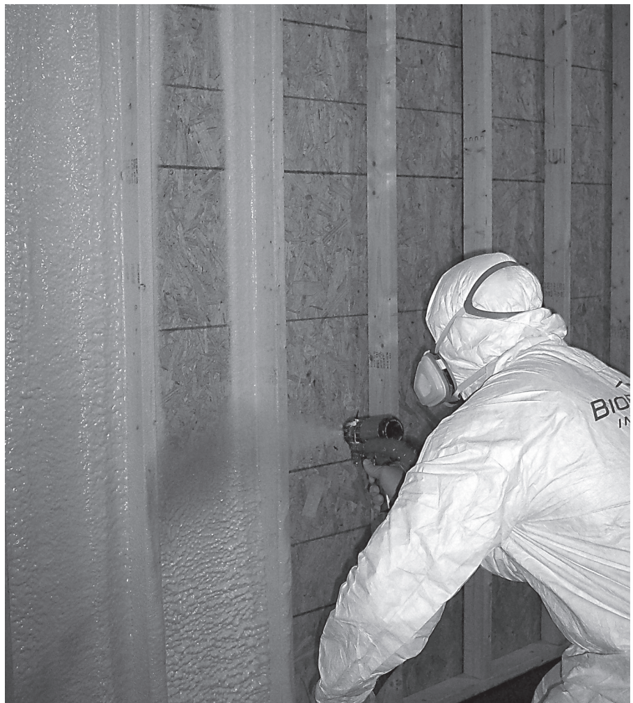
Figure 6.8 Spray foam insulation helps to seal any leaks of conditioned air to the exterior environment, thus optimizing energy use. Photo courtesy of BioBased Technologies
