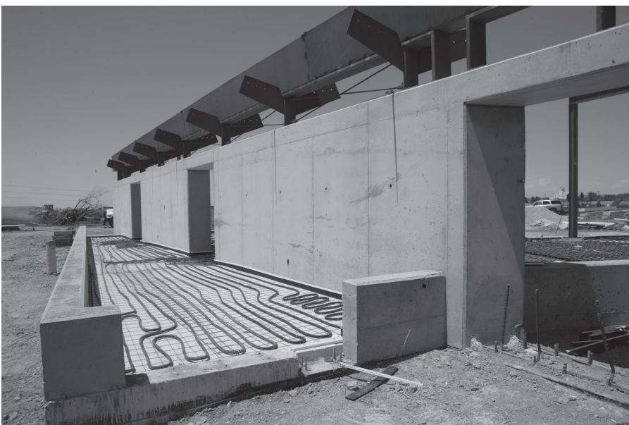
Figure 6.3 The Wetland Discovery Point building at Utah State University utilizes a trombe wall to capture heat from the sun, as well as radiant heat flooring to increase the energy efficiencies of the project.
