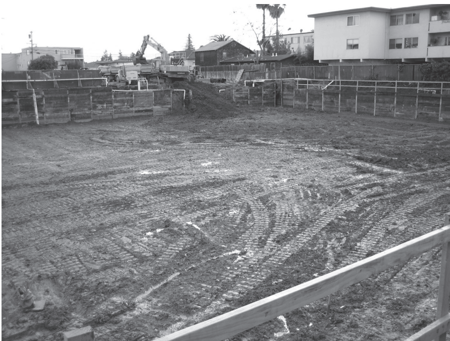
Figure 4.2 Villa Montgomery Apartments, a remediation project in Redwood City, California, by Fisher-Friedman Associates, earned LEED Gold certification, for compliance with multiple Sustainable Sites strategies, including brownfield site selection and remediation.
