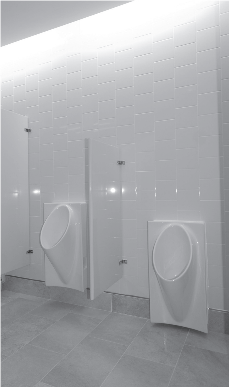
Figure 5.2 Waterless urinals help to reduce the indoor water consumption. Photo courtesy of SmithGroup, Inc.
