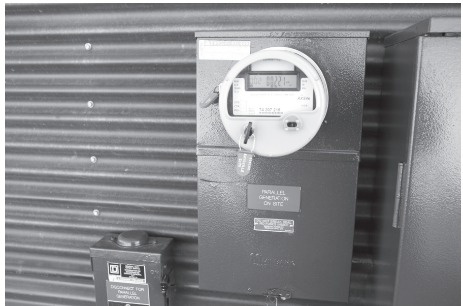
Figure 6.12 Metering utilities to monitor consumption helps building owners and facility managers ensure that the building is functioning properly. Photo courtesy of Gary Neuenswander, Utah Agricultural Experiment Station
