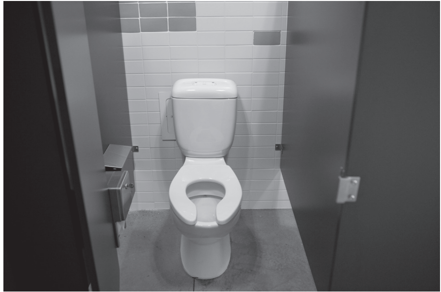
Figure 4.15 Using dual-flush toilets reduces the need for potable water at the Utah Botanical Center’s Wetland Discovery Point building. Photo courtesy of Gary Neuwander, Utah Agricultural Experiment Station
