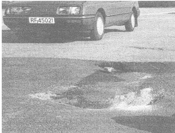
Fig. 9 - Example of Pavement Settlement due to Voids
