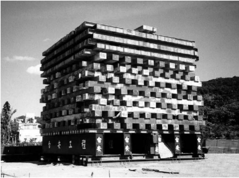
Figure 8.36 Pile load test using the Kentledge method. (Courtesy of DECL, Taipei, Taiwan.)
