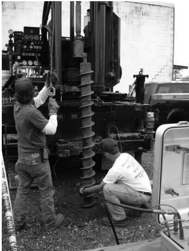
Figure 3.9 Hollow stem auger in operation, Washington, DC, USA. (Courtesy of An-Bin Huang, Hsinchu, Taiwan.)
