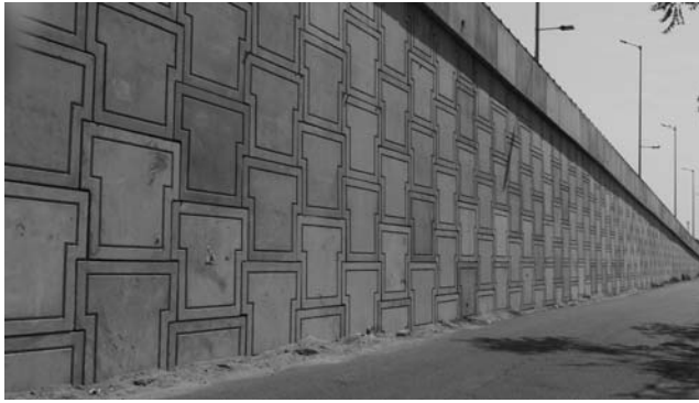
Figure 5.21 A geosynthetic reinforced soil-retaining wall in Jodhpur, India. (Courtesy of An-Bin Huang, Hsinchu, Taiwan.)
