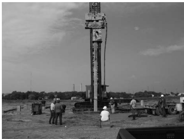
Figure 8.3 Driving of a steel H pile with a vibratory driver in Houston, Texas, USA. (Courtesy of Dr. Kenneth Viking, Stockholm, Sweden.)
