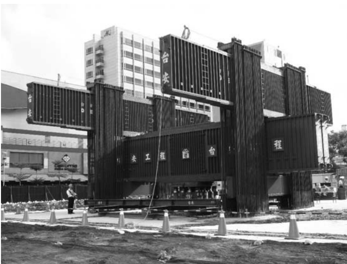
Figure 8.35 Pile load test using a reaction frame with 75,000 kN capacity. (Courtesy of DECL, Taipei, Taiwan.)
