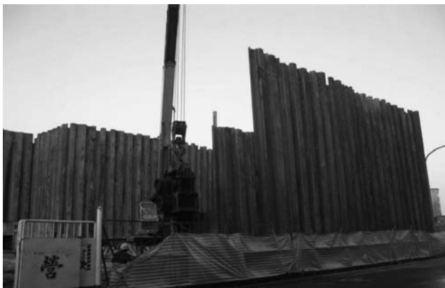
Figure 5.22 Field installation of a sheet pile wall. (Courtesy of Trinity Foundation Engineering Consultants, Co. Ltd., Taipei, Taiwan.)
