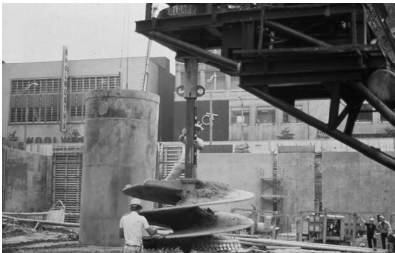
Figure 8.20 Typical power auger used to advance the borehole. (Courtesy of An-Bin Huang, Hsinchu, Taiwan.)
