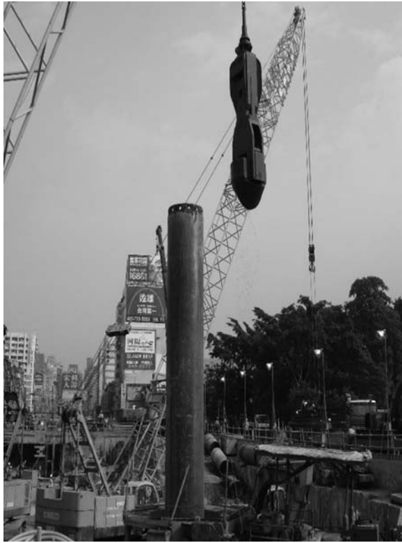
Figure 8.26 Field operation of an oscillator rig used to insert casing and a hammer grab. (Courtesy of An-Bin Huang, Hsinchu, Taiwan.)
