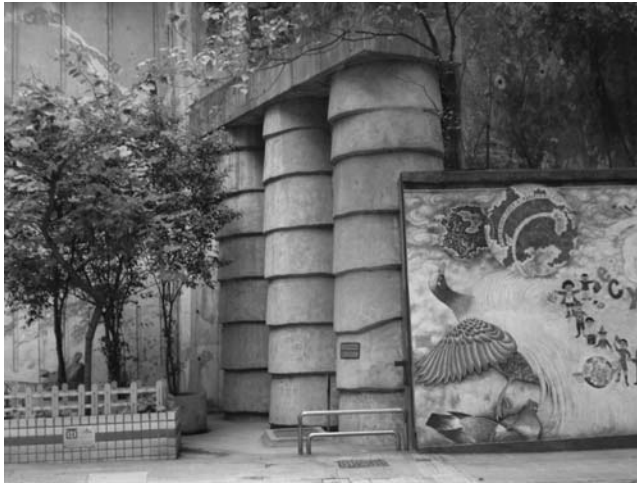
Figure 7.27 Bored piles for slope stabilization in Midlevel, Hong Kong. (Courtesy of An-Bin Huang, Hsinchu, Taiwan.)
