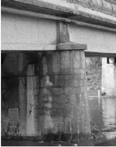
3.7 Cracking pattern in a bridge suffering from internal sulfatic attack (from Germain, 2008).
