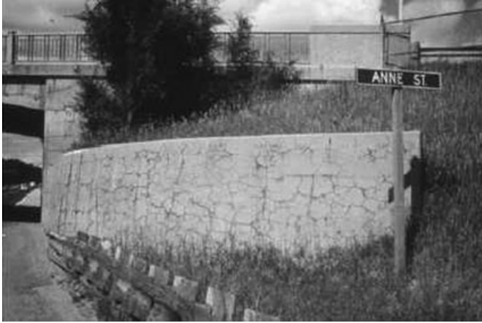
3.5 Surface crack network owing to AAR (from Balayssac, 2005).
