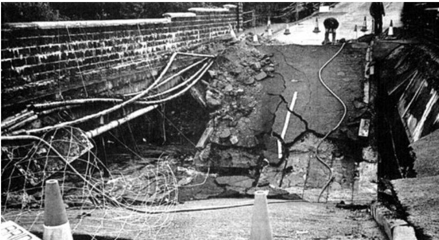
1.6 Collapse of the Ynys-y-Gwas bridge led to a ban on grouted tendons. 17
