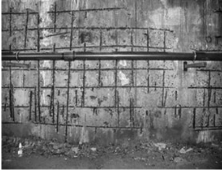
3.2 Consequences of corrosion in a concrete wall (from Balayssac, 2005).
