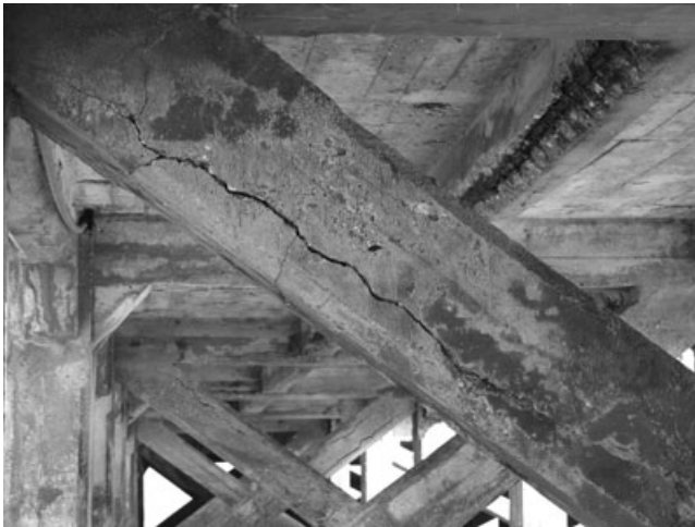
3.3 Cracking and spalling owing to corrosion in a marine environment.
