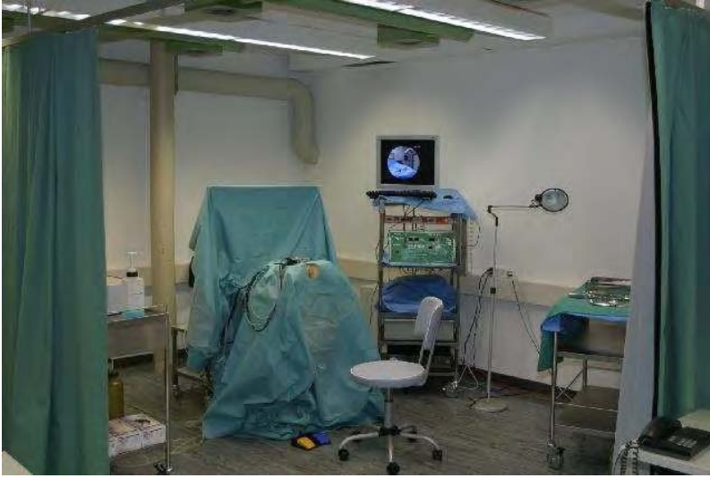
Figure 1. View of the complete OR.
