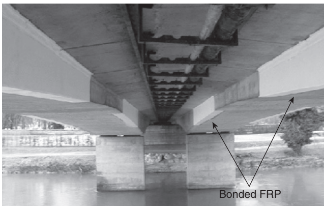
20.11 View of the bridge under consideration; FRP repaired zones correspond to the white parts on the girders.
