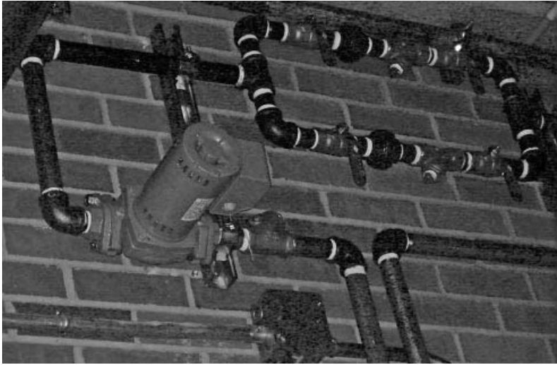
Figure 3.5 Pipes and an in-line pump mounted on brackets
