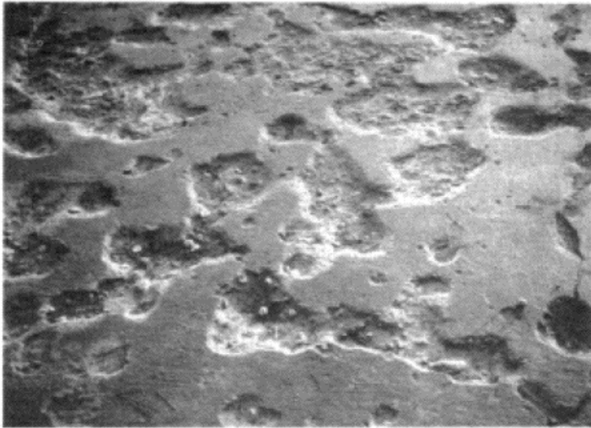
Fig. 5.12. Concrete dock surface spalled and eroded by salt crystallization from evaporated seawater puddles (courtesy: J.Figg).
