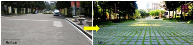
Fig.22:The original impermeable pavement reform to new permeable pavement with structural support
