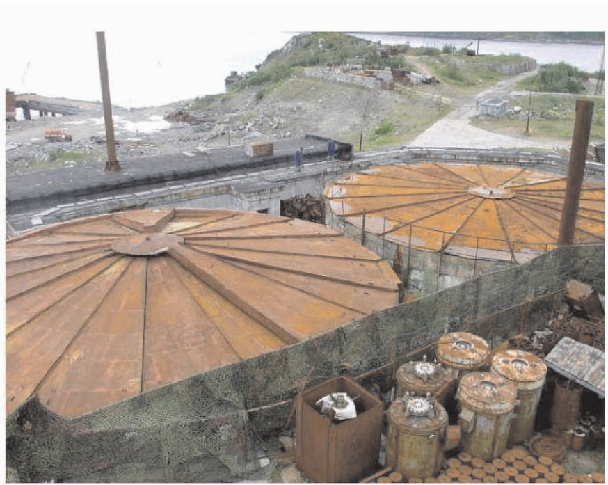
Figure 1. Dry Storage Units 2,3 (facilities 2A and 2B)
