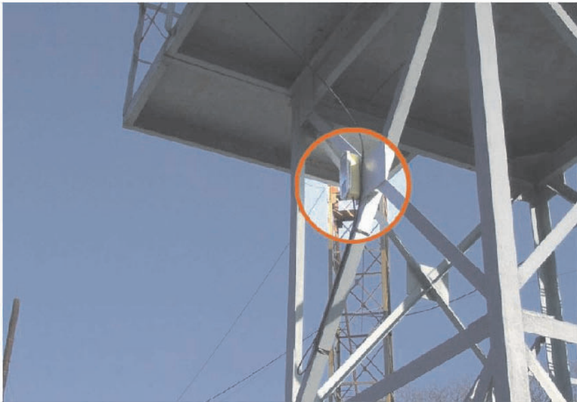
Figure 5. Exposure dose rate sensor at DalRAO's temporary storage facility for RC units (Razboinik Bay)
