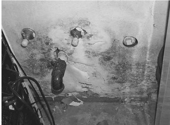
Figure 7.1 Typical mold patterns on walls. (Courtesy of Aerotech Laboratories, Phoenix, AZ.)
