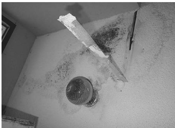
Figure 7.6 Mold on ceiling (be sure to check electrical fixtures also). (Courtesy of Aerotech Laboratories, Phoenix, AZ.)
