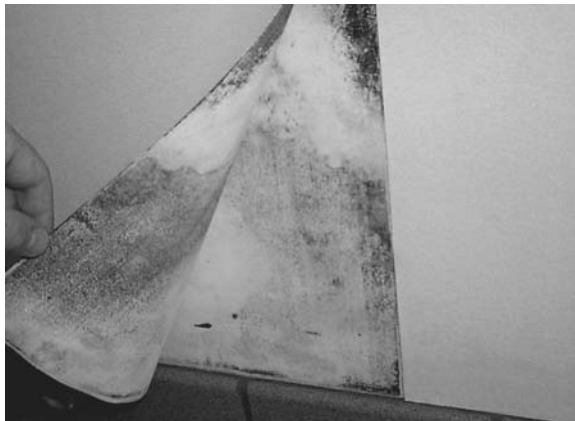
Figure 7.5 Mold under wallpaper. (Courtesy of Aerotech Laboratories, Phoenix, AZ.)
