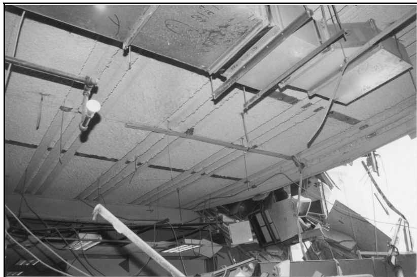
Figure 9b. Interior damage at tenant levels 22 and 21—underside of level 22 slab looking northwest.
