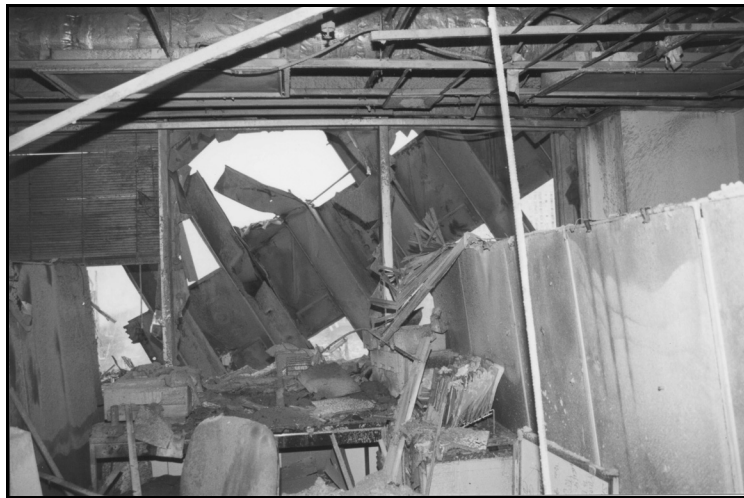
Figure 13b. Building damage at tenant level 9— view of inside face of tower 2 façade element.
