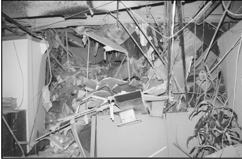
Figure 13a. Building damage at tenant level 9— complete destruction of one zone of the building.
