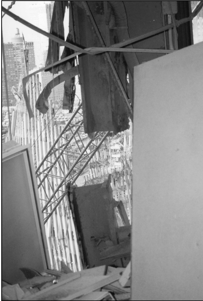
Figure 11a. Fractured column on line D from tenant levels 18 and 17—view at level 18.
