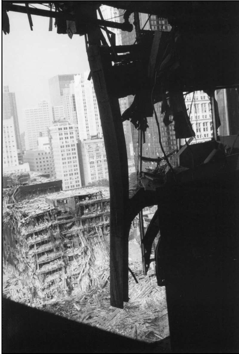
Figure 11b. Fractured column on line D from tenant levels 18 and 17—view at level 17.
