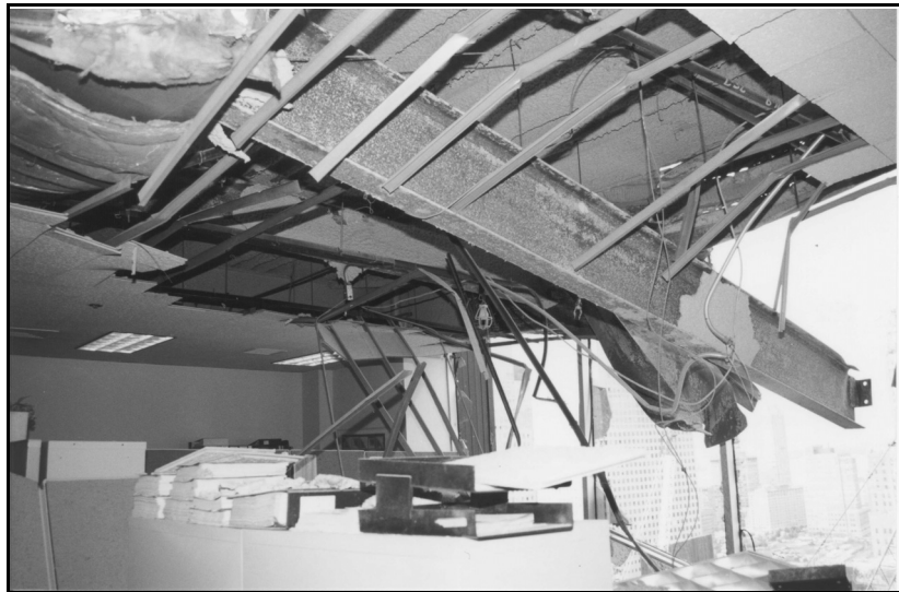
Figure 9a. Interior damage at tenant levels 22 and 21—underside of level 23 slab looking northwest.
