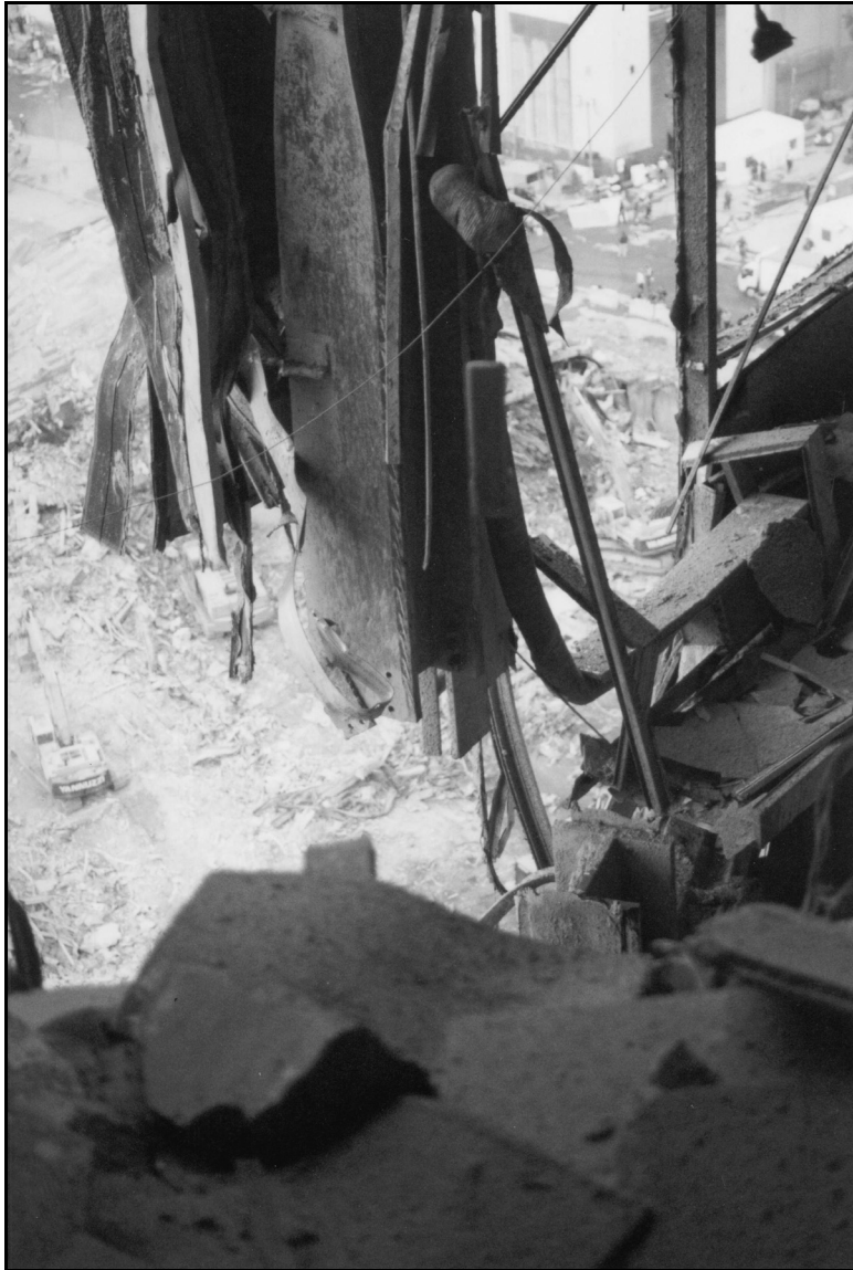
Figure 10d. Interior damage photographs from tenant level 19— failed column immediately above level 18.
