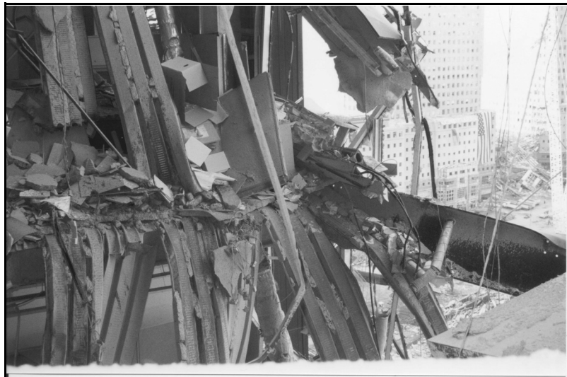
Figure 10b. Interior damage photographs from tenant level 19— floor framing on line 8 between lines C and D.
