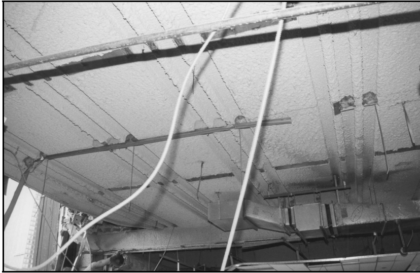
Figure 9c. Interior damage at tenant levels 22 and 21—underside of level 22 slab looking northeast.
