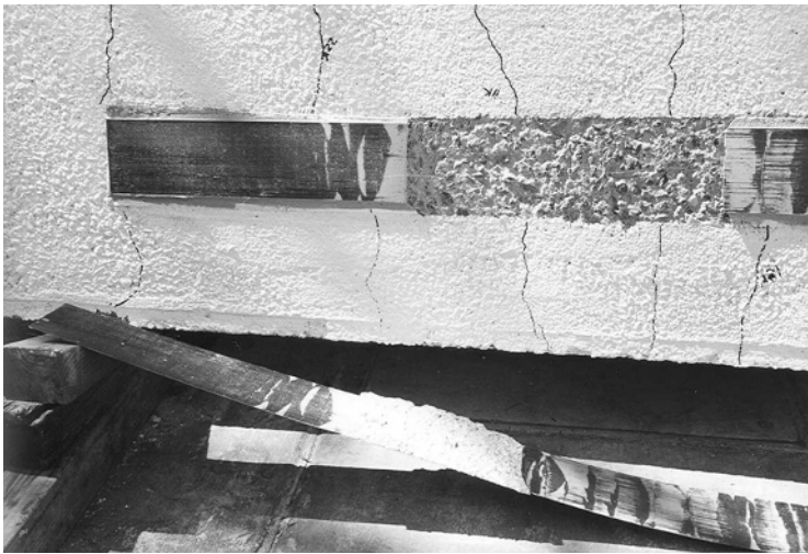
5.4 Close-up showing splitting within the prefabricated strip.
