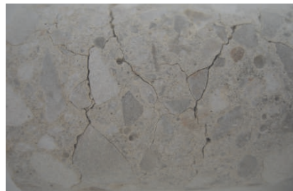
Fig. 4. Photograph of a small cylinder of concrete CEMII/59 subjected to cycles of immersion-drying at 60°C
