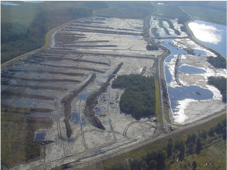
Fig. 4.7 De-mucking scene of the northern flow train shows dewatering of rows of muck, prior to removal
