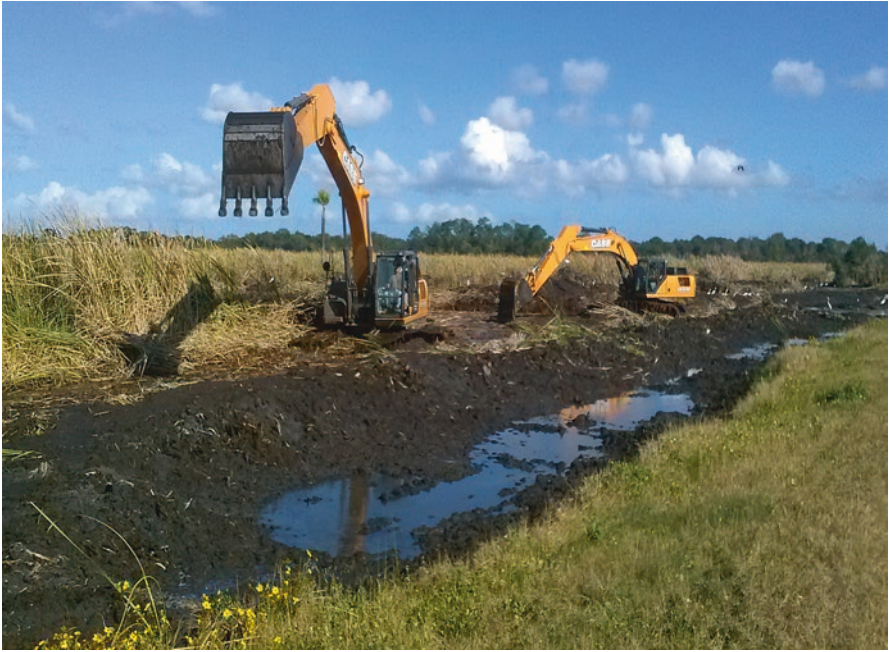
Fig. 4.6 Excavators install ditches to help dewater wetland muck before windrowing and muck removal
