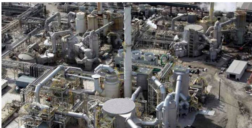
Sulfuric acid plant [DSD Chemtech]
