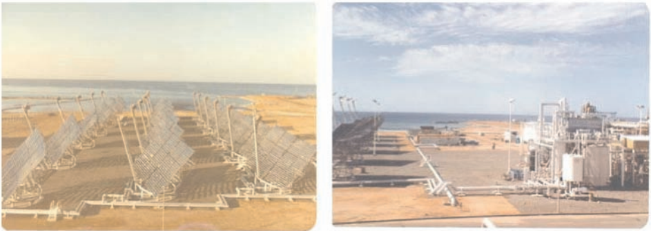
Figure 6: Pilot Solar Thermal Desalination Plant in Saudi Arabia
